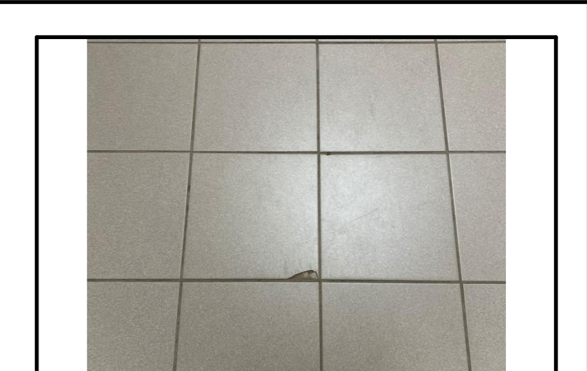
PCT DAMAGE - CORRIDOR 106
