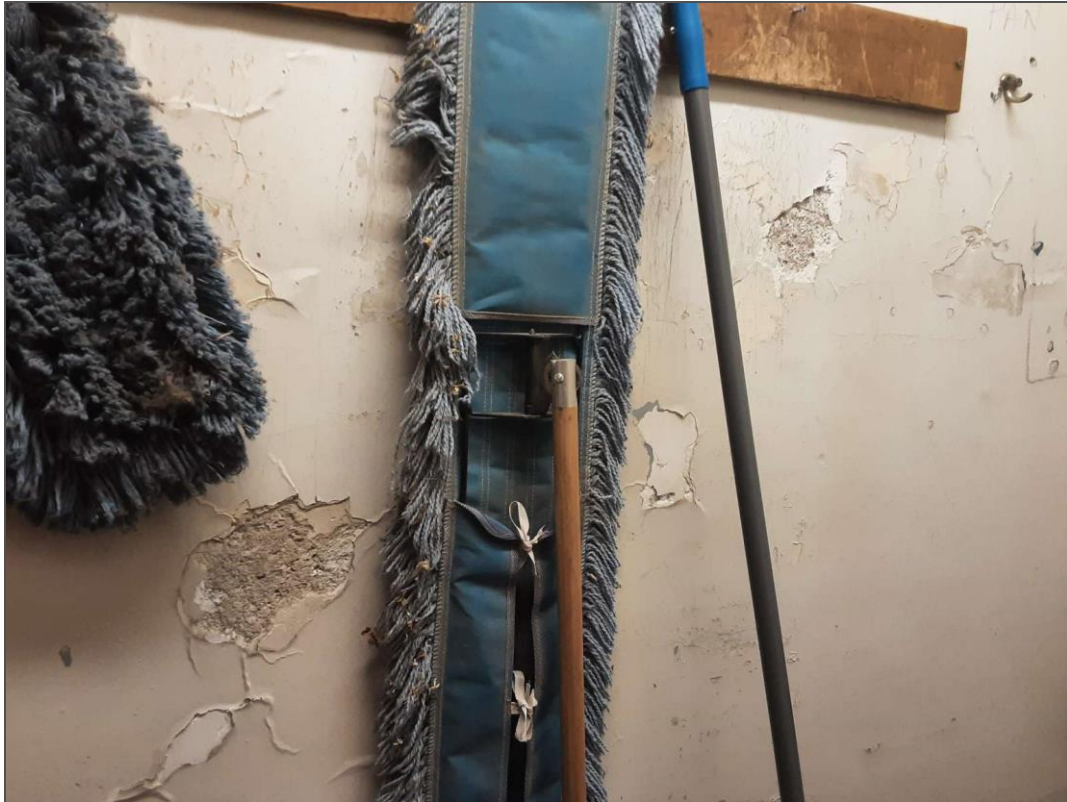
S0029 - Asbestos-Containing Smooth Plaster in Poor Condition, Closet (Location #: 133).
