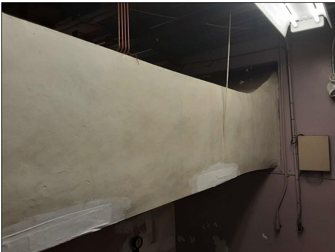
S0038 - Asbestos-Containing Parging Cement Duct Insulation, Fan Room (Location #: 264).
