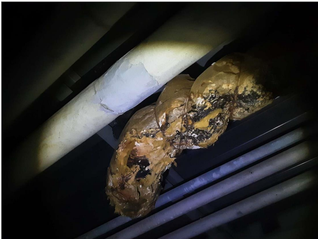
S0018 - Asbestos-Containing Sweatwrap Insulation in Poor Condition, Fan Room (Location #: 264).
