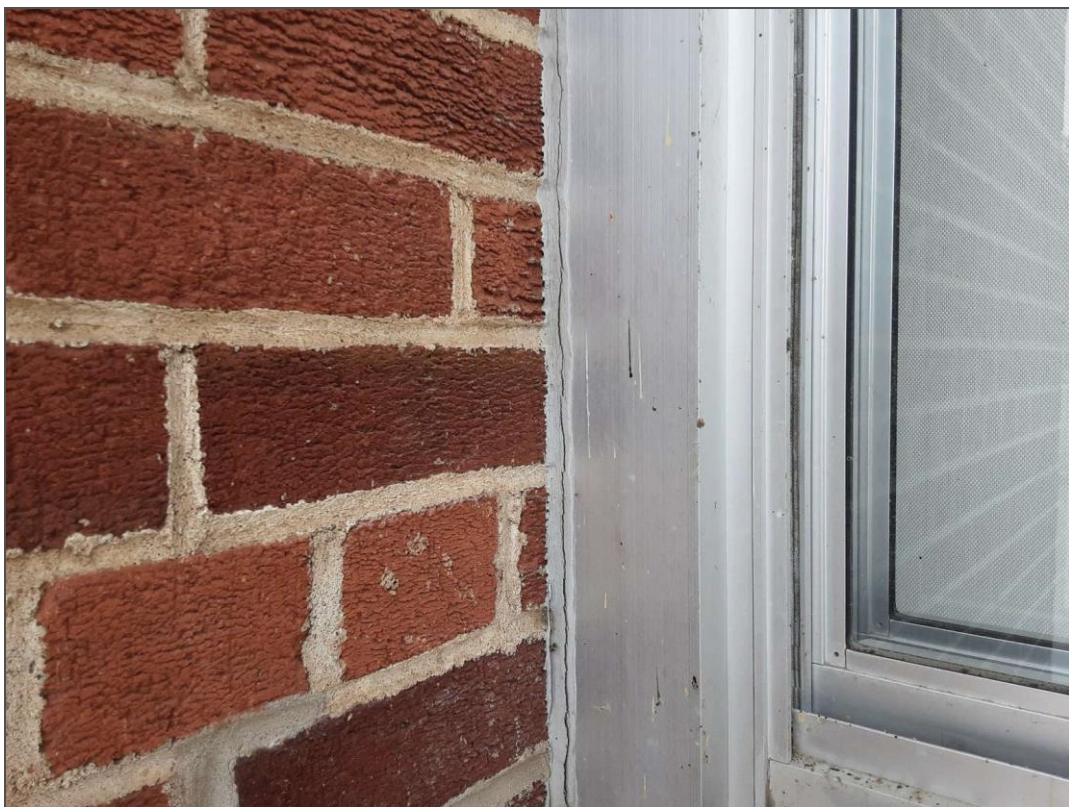
S0013 – Asbestos-Containing Soft Grey Window Caulking, Exterior - Original Building (Location #: 500).
