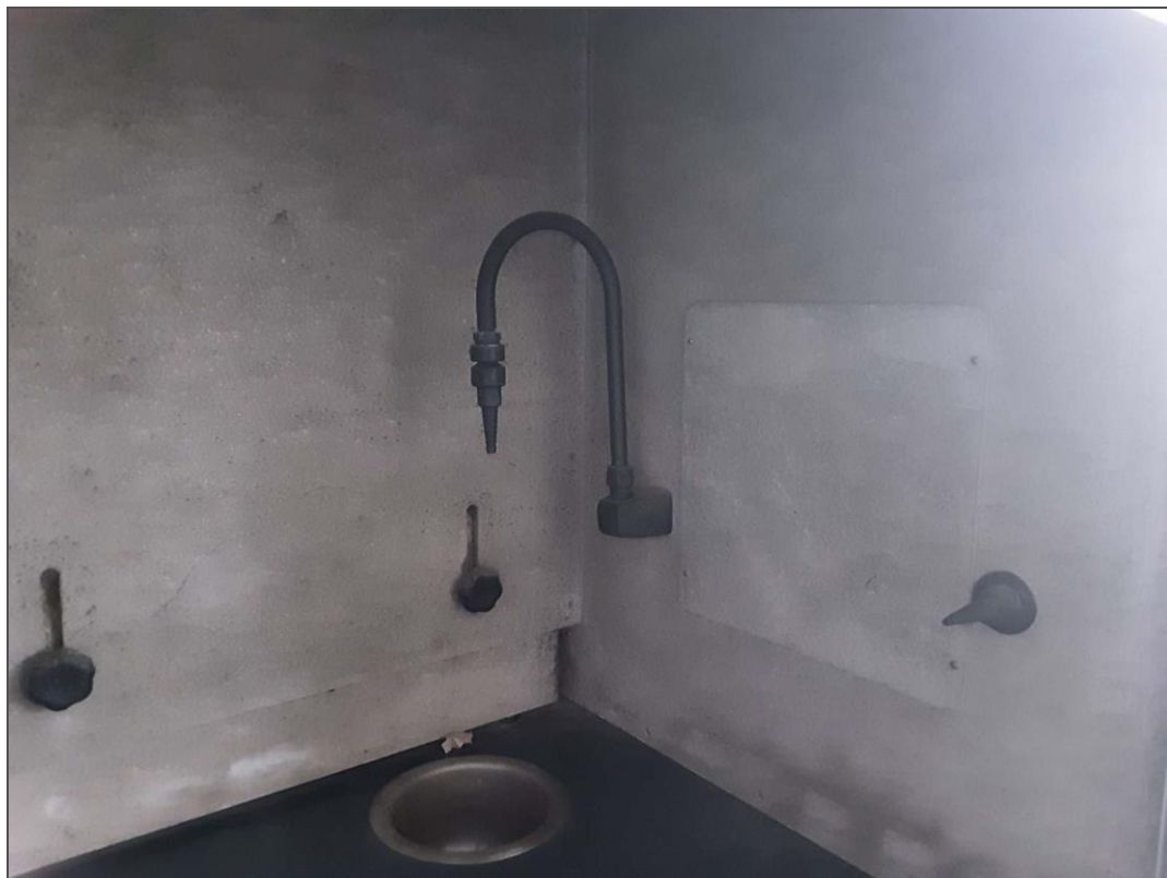
V9500 – Presumed Asbestos-Containing Transite Board within Fume Hood, Classroom (Location #: 201).
