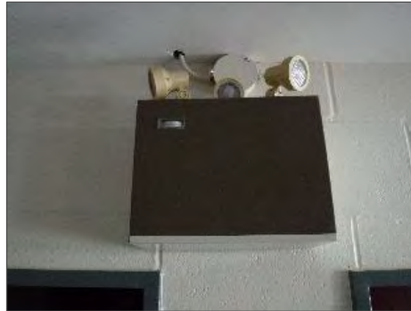
Emergency light containing lead-acid batteries.
