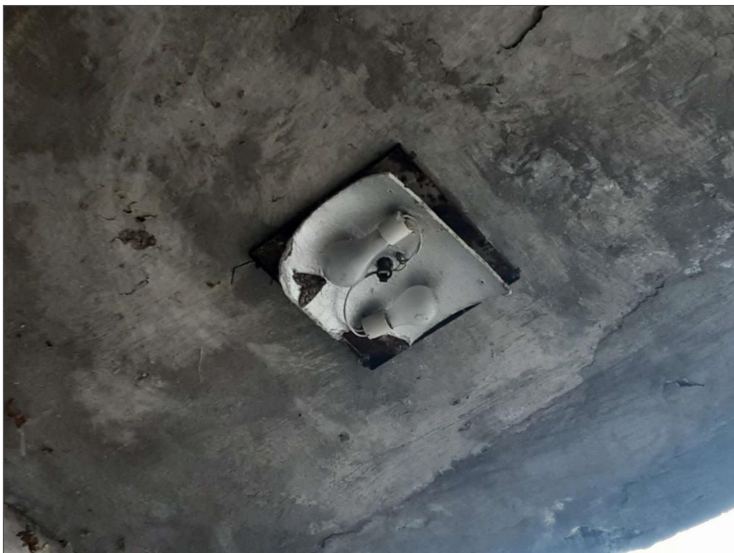
S0042 - Asbestos-Containing Paper Heat Shield, Corridor (Location #: 163).
