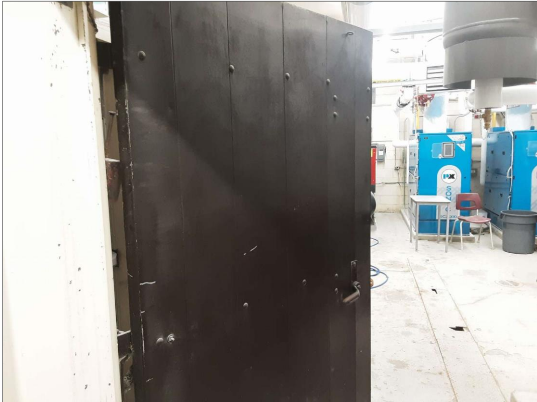
V9500 – Presumed Asbestos-Containing Insulation within Fire Rated Door, Electrical Room (Location #: 140).
