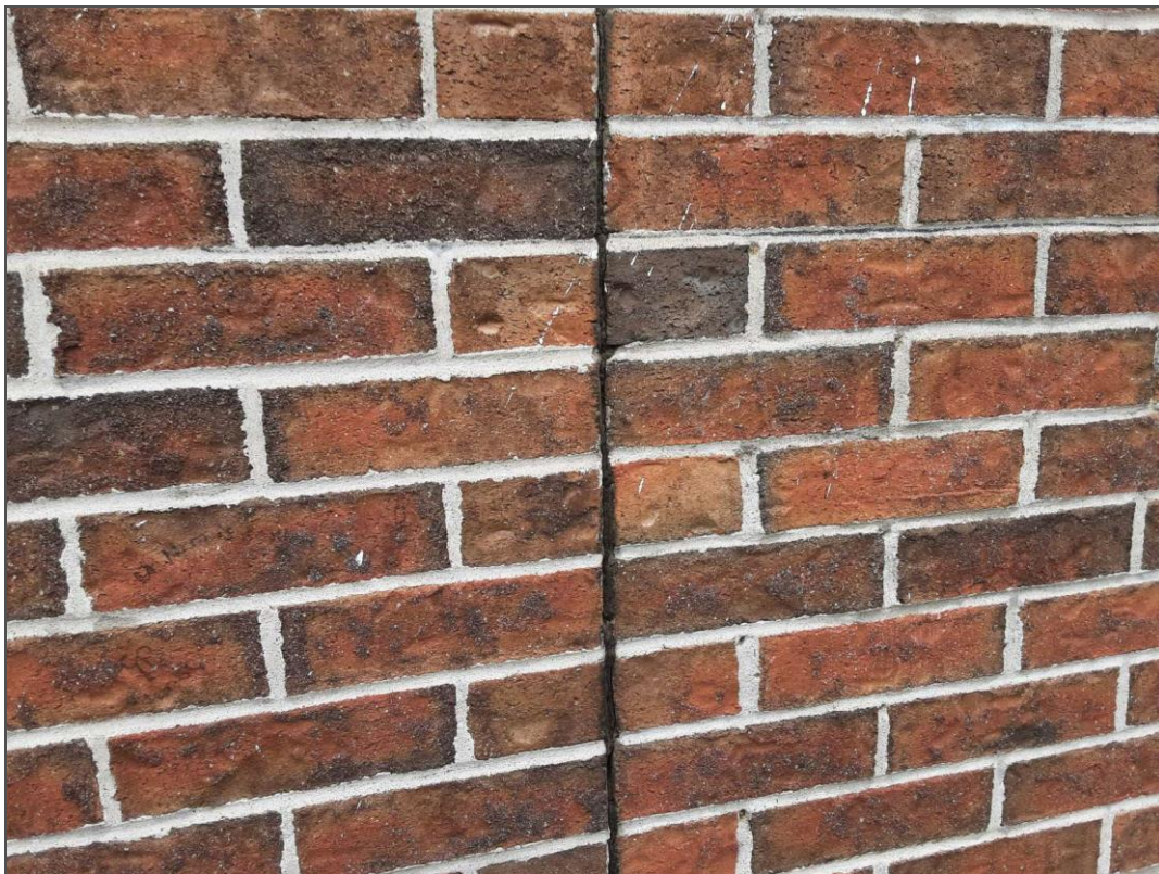
S0009 – Asbestos-Containing Soft Black Expansion Joint Caulking, Exterior - Original Building (Location #: 500).
