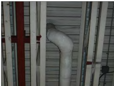
Asbestos-containing parging cement insulation present on pipe fitting, in good condition
