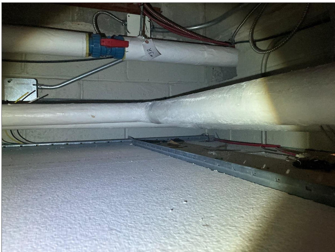
S0021 - Asbestos-Containing Aircell Insulation, Corridor (Location #: 162).
