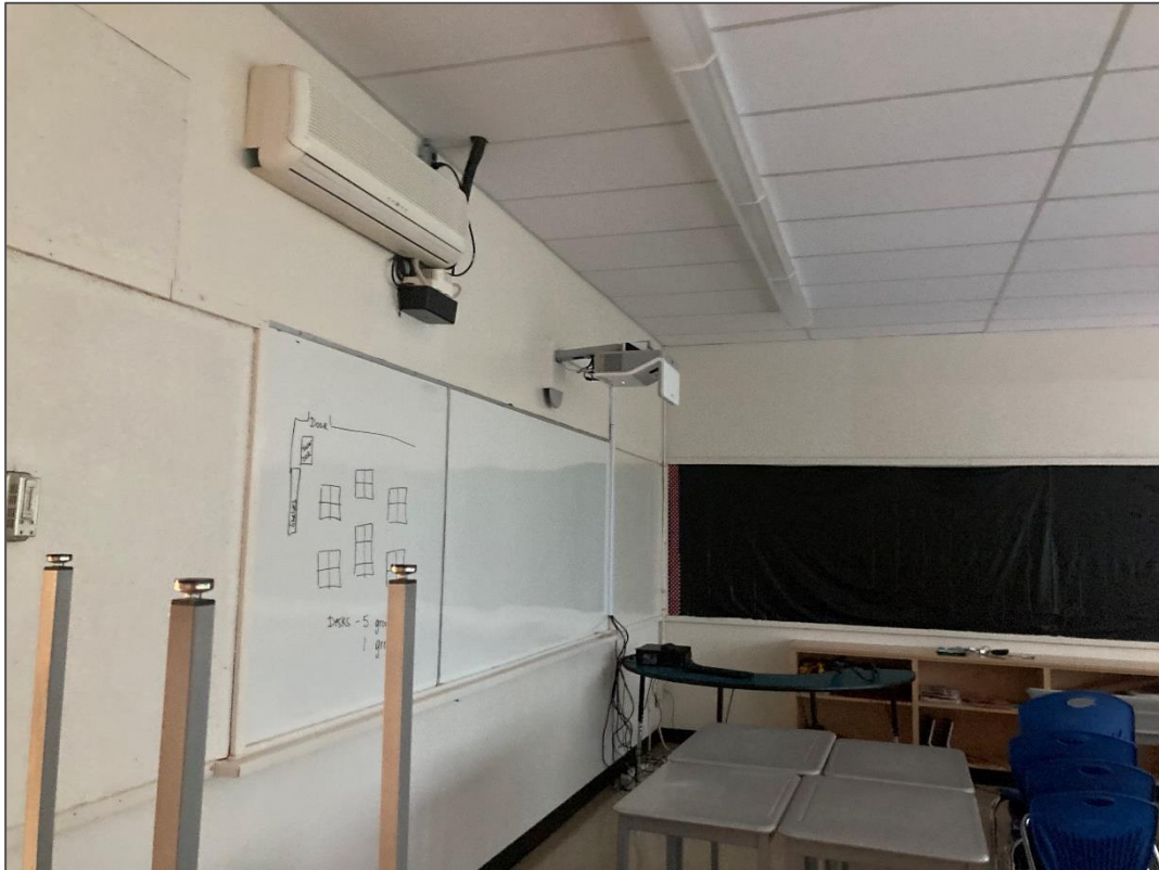
S0050 – Asbestos-Containing Plaster, Classroom (Location #: 202).
