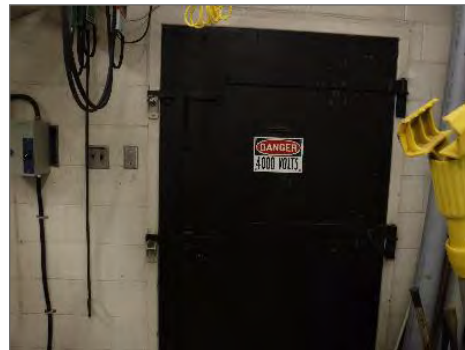
Suspected asbestos-containing insulation within the core of the fire rated door for room 140.
