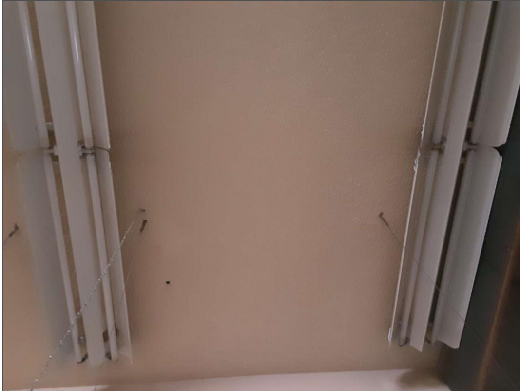
S0045 - Asbestos-Containing Texture Coat Ceiling, Classroom (Location #: 1182).
