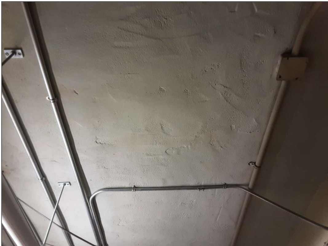
S0048 - Asbestos-Containing Rough Plaster Ceiling, Basement (Location #: 18).
