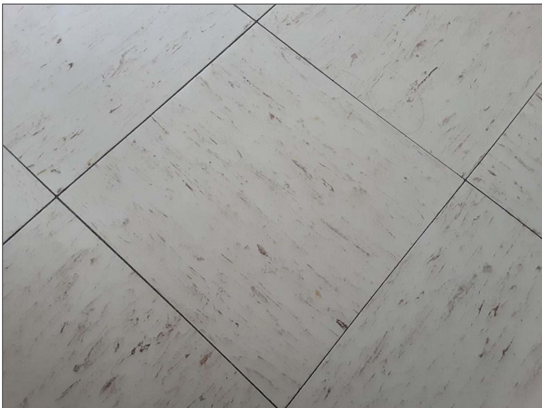
S0028 - Asbestos-Containing 12"x12" Beige Vinyl Floor Tiles with Burgundy Streaks, Classroom (Location #: 101).
