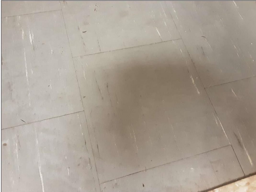
S0024 - Asbestos-Containing 9"x9" Dark Grey Vinyl Floor Tiles with White Streaks and Mastic, Closet (Location #: 1141).
