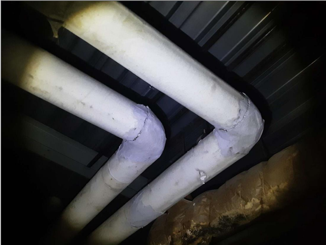
S0019 - Asbestos-Containing Parging Cement Insulation in Poor Condition, Fan Room (Location #: 264).
