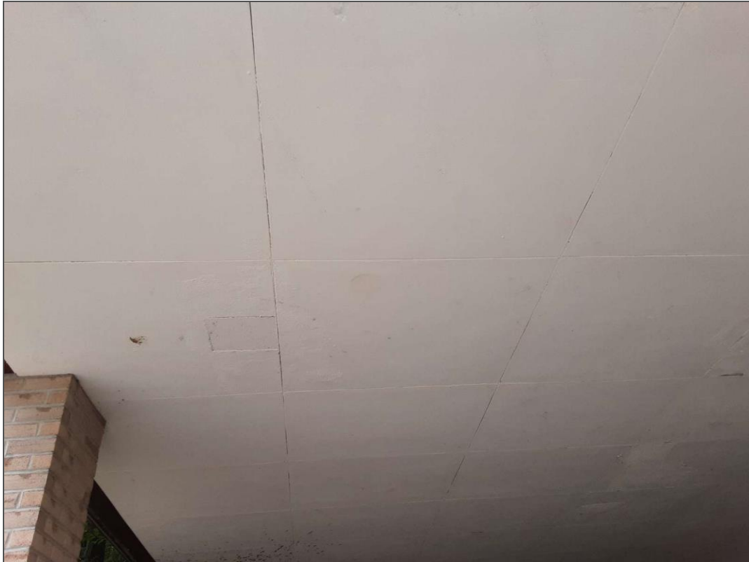
S0012 – Asbestos-Containing Stucco Canopy, Exterior - 1962 Addition (Location #: 502).
