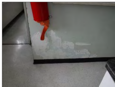
Peeling and flaking mint paint present in Room 101A.
