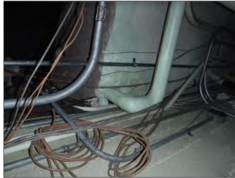
Asbestos-containing Aircell pipe present throughout the building
