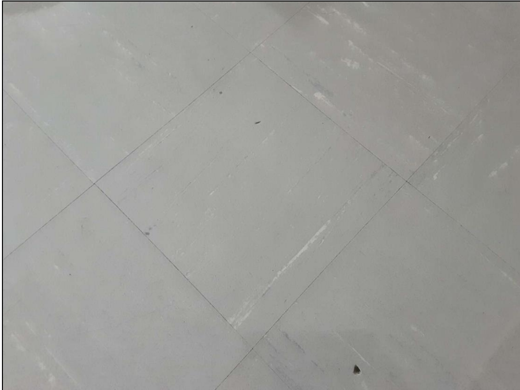
S0017 – Asbestos-Containing 9"x9" Light Grey Vinyl Floor Tiles with White Streaks and Mastic, Classroom (Location #: 120).
