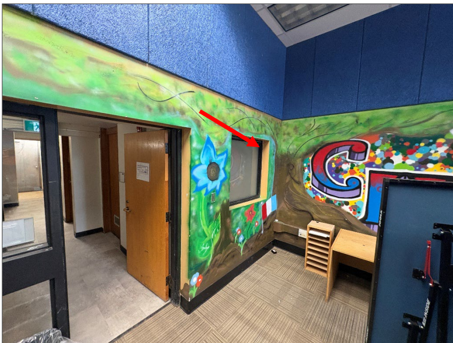
Photo 2: Non-lead based black paint on interior window frame.
