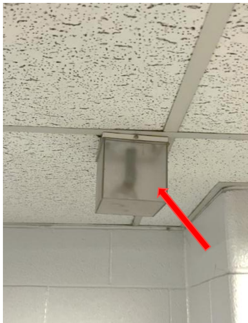
Photo 4. Representative view of assumed lead-containing batteries associated with emergency lighting system observed in Room 127.
