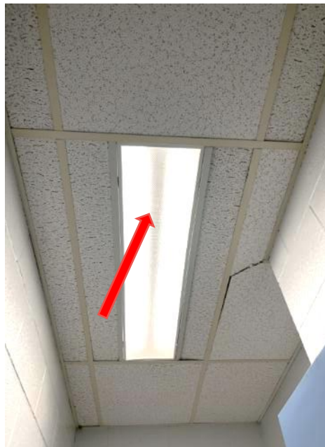
Photo 2. Representative view of assumed mercury-containing fluorescent light tubes and assumed PCB-containing light ballasts observed in the Corridor.
