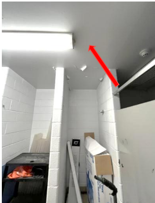
Photo 2. Representative view of low-level lead paint described as white applied to drywall ceiling observed in Room 127.
