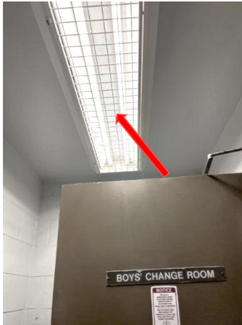
Photo 3. Representative view of light fixture equipped with LED light tubes observed in Room 127.
