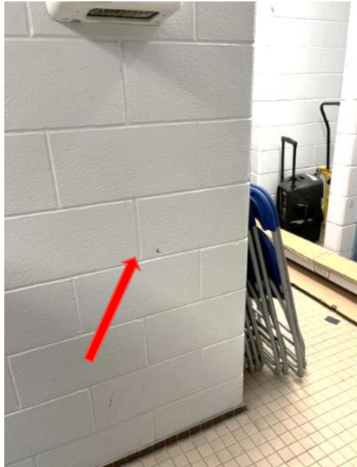
Photo 1. Representative view of low-level lead white paint applied to concrete block wall observed in Room 127.
