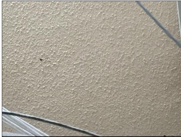
Asbestos-containing texture finish on the ceilings in Room 118B.
