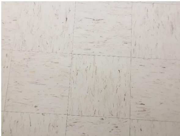
Asbestos-containing 12" beige vinyl floor tiles with burgundy streaks (VT5).
