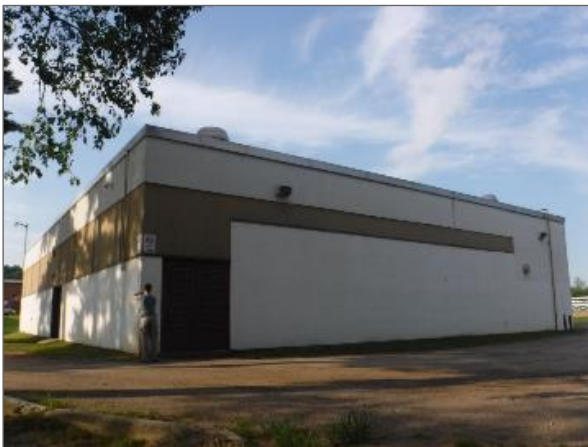
Asbestos-containing stucco present on the exterior walls of the 1959, 1962 and 1966 additions.
