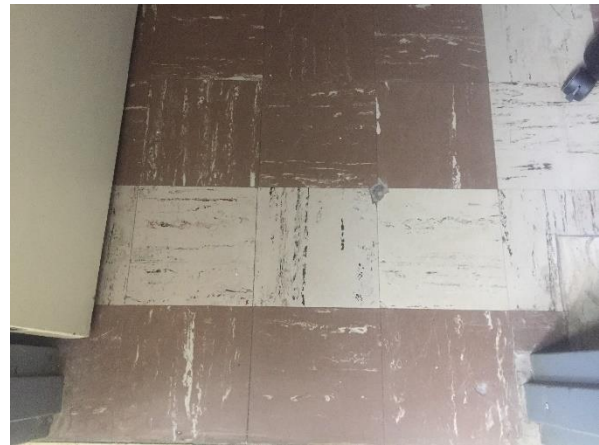
Asbestos-containing 9" vinyl floor tiles brown with white streaks and white with brown streaks and mastic (VT8).
