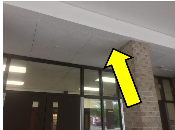
Asbestos-containing stucco panels present on the underside of the southeast entrance of the 1962 addition (under the music room 214).
