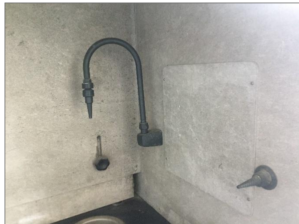
Presumed asbestos-containing Transite board within fume hood.
