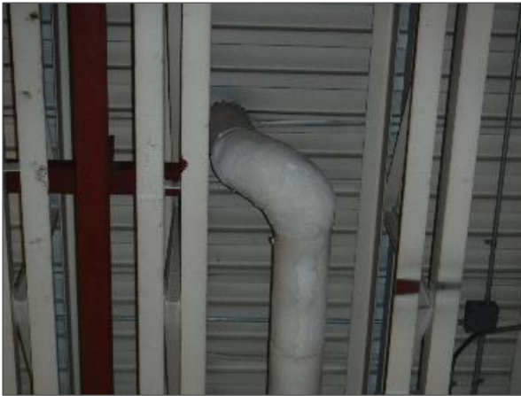
Asbestos-containing paring cement insulation present on pipe fitting, in good condition
