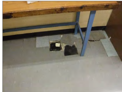
Loose and delaminating asbestos-containing 9" dark grey vinyl floor tiles with white streaks (VT3) in room 114A.
