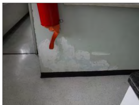
Peeling and flaking mint paint present in Room 101A.
