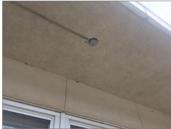
Non-asbestos grey stucco present between windows and on the underside of the soffits of the 1947 original building.
