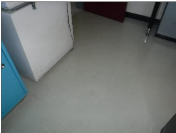
Asbestos-containing 9" light grey vinyl floor tiles with white streaks and mastic (VT1).
