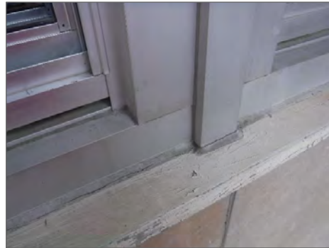
Asbestos-containing grey, soft exterior window caulking on the 1947 original building and 1962 addition.
