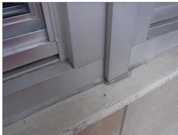
Asbestos-containing grey, soft exterior window caulking on the 1947 original building and 1962 addition.
