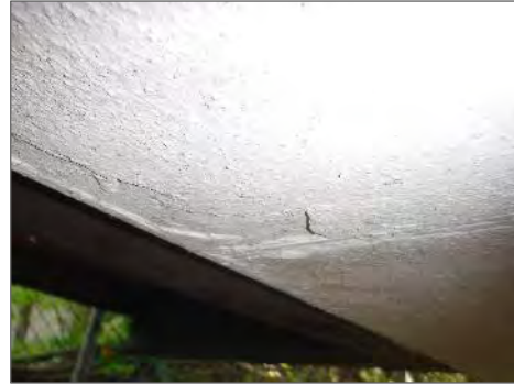
Asbestos-containing stucco panels present on the underside of the southeast entrance of the 1962 addition (under the music room 214).
