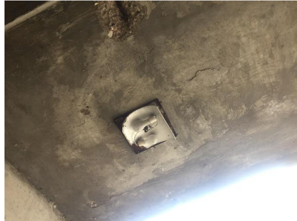
Asbestos-containing paper heat shield present within two exterior incandescent light fixtures at the entrance to Corridor 163.
