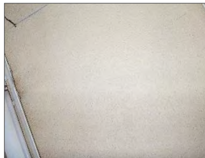
Asbestos-containing texture finish on the ceilings in Room 118B.
