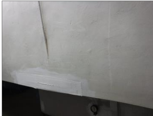
Asbestos-containing paring cement present under canvas jacketing on ducts in room 164.
