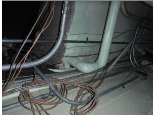
Asbestos-containing Aircell pipe present throughout the building
