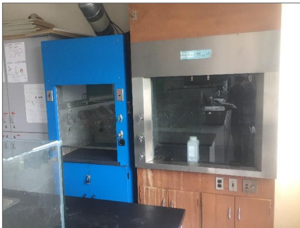
Fume hoods with presumed asbestos-containing Transite board in Room 201
