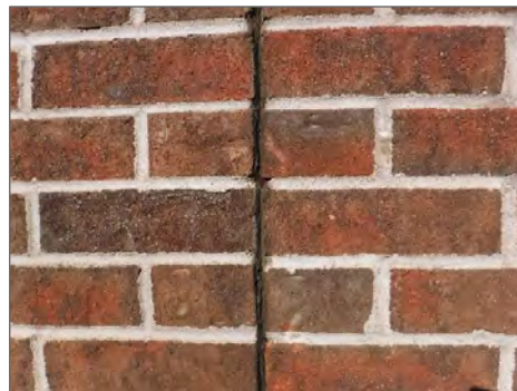
Asbestos-containing black, soft exterior expansion joint caulking on the 1947 original building.
