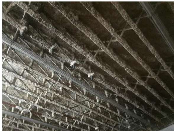
Non-asbestos spray-applied fireproofing in gymnasium 158.
