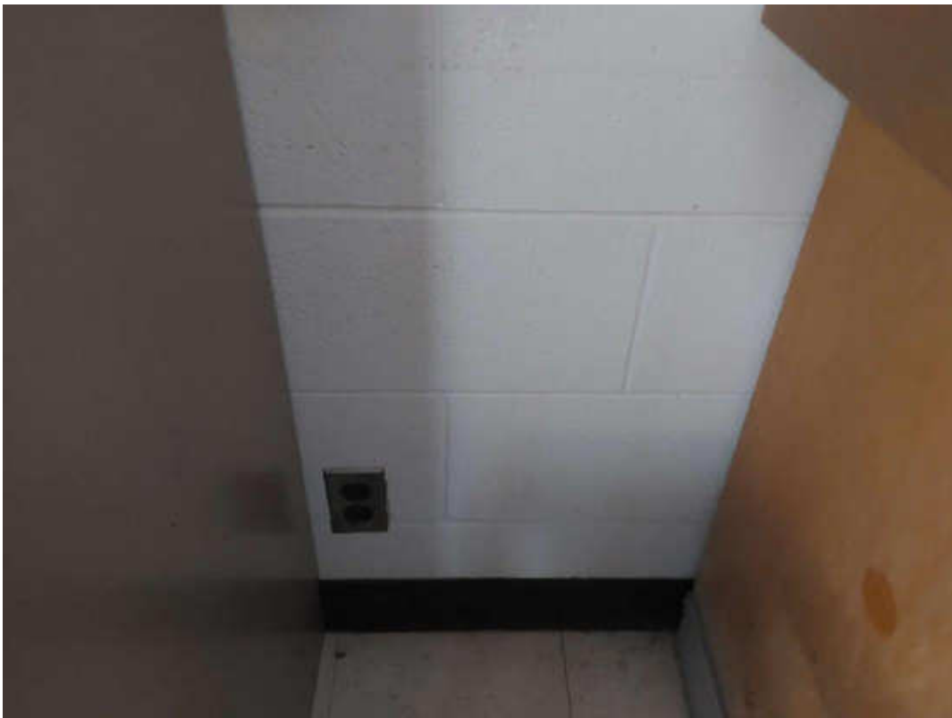
V9000 (Confirmed Asbestos), Wall, Vermiculite Investigation, Offices (Location #: 30) Vermiculite found
