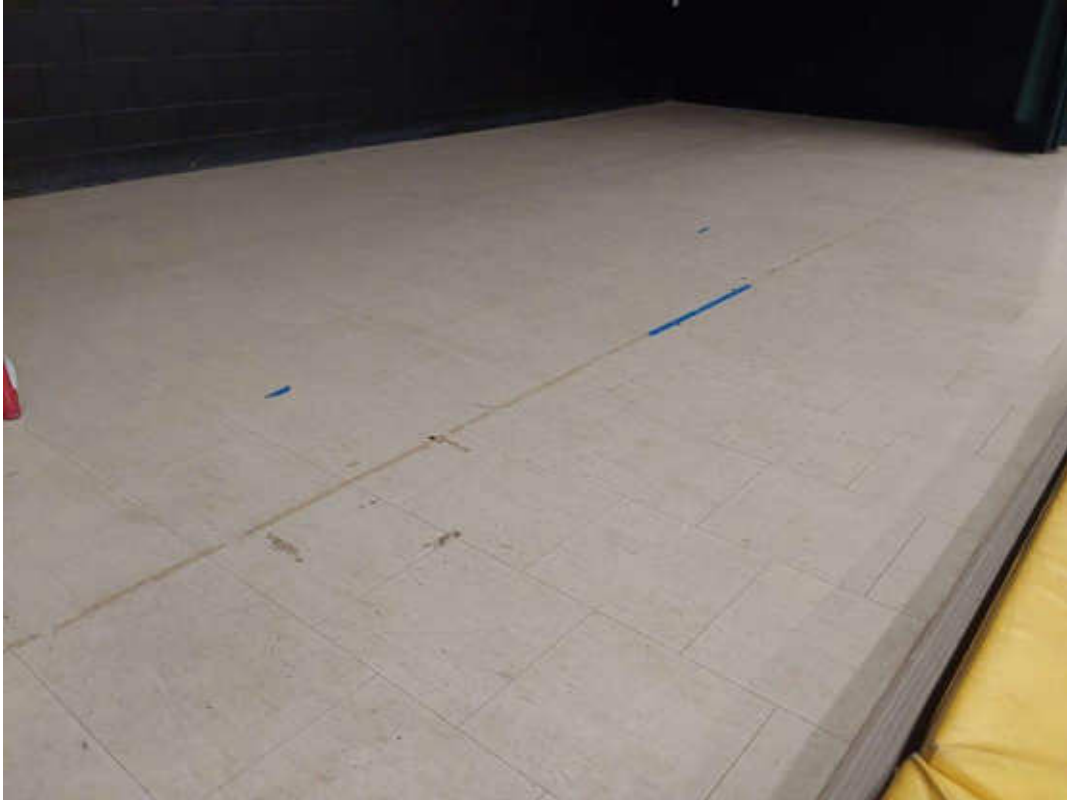
V0020 (Confirmed Asbestos), 12 x 12 off-white with brown streaks, Floor, Vinyl Floor Tile and Mastic, Gym (Location #: 1) Stage floor, Mastic is presumed to contain asbestos
