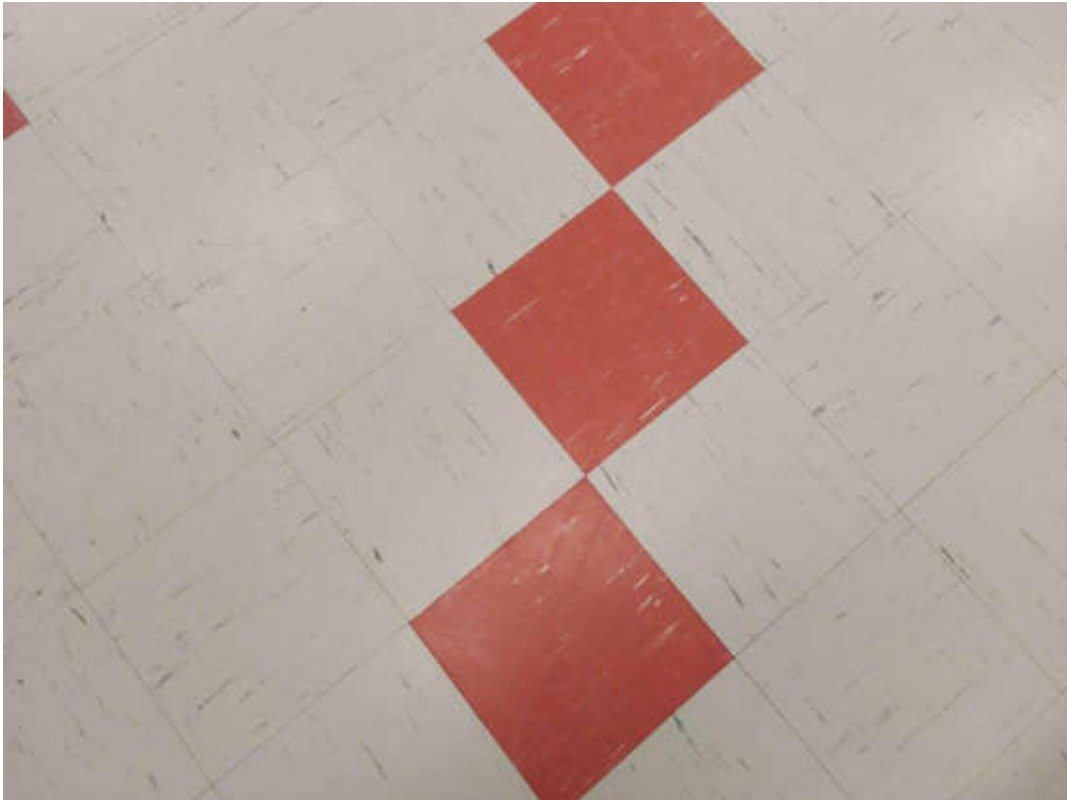
S0018 (Confirmed Asbestos), 9 x 9 red with white streaks, Floor, Vinyl Floor Tile and Mastic, Room 1 (Location #: 4) Mastic is presumed to contain asbestos
