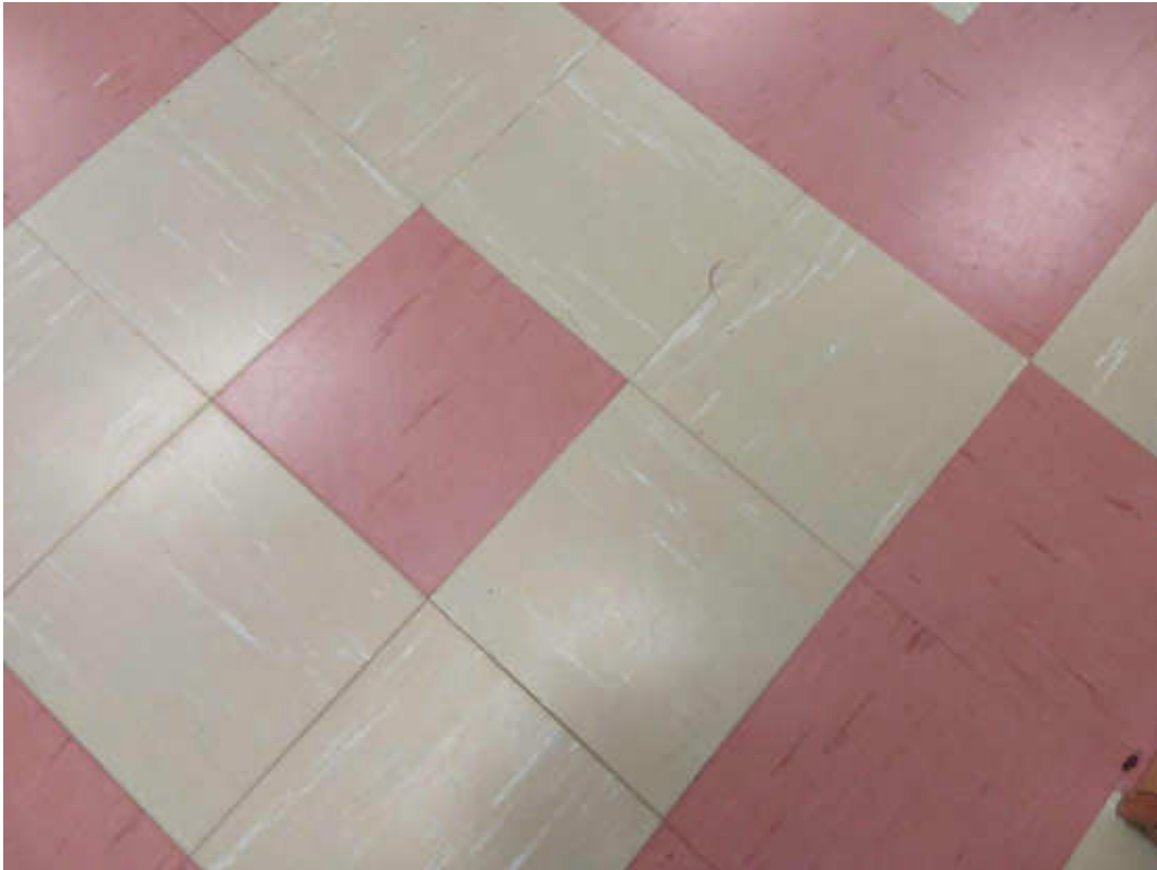
V0002 (Confirmed Asbestos), 9 x 9 beige with white streaks, Floor, Vinyl Floor Tile and Mastic, Room 3 (Location #: 5) Mastic is presumed to contain asbestos
