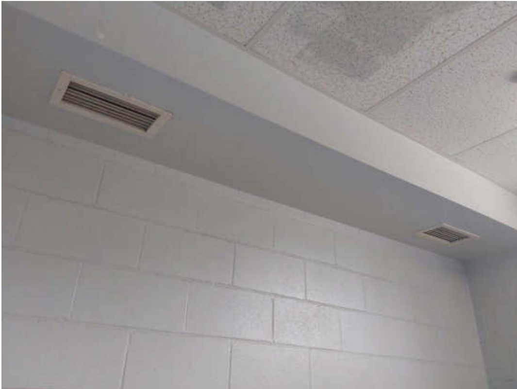
V0028 (Confirmed Asbestos), Ceiling, Drywall and joint compound, Men's Washroom (Boys) (Location #: 12)
