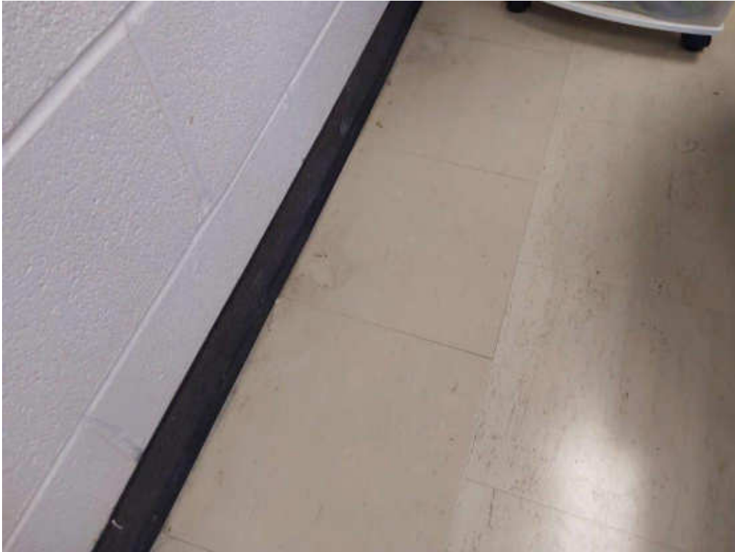
V9500 (Presumed Asbestos), 12 x 12 beige with brown flecks, Floor, Vinyl Floor Tile and Mastic, Classroom 115 (Location #: 43) Mastic is confirmed to contain asbestos
