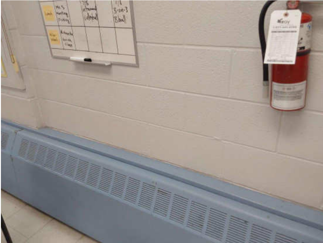
V9500 (Presumed Asbestos), Wall, Vermiculite/concrete block walls, Staff Room (Location #: 16)
