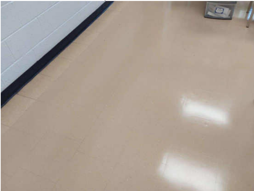
S0019 (Confirmed Asbestos), 12 x 12 orange, Floor, Vinyl Floor Tile and Mastic, Classroom 105 (Location #: 27) Mastic is confirmed to contain asbestos
