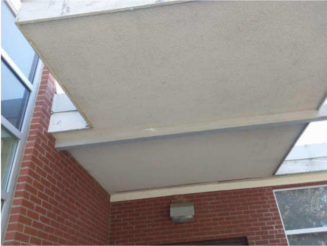
V9000 (Confirmed Asbestos), Wall, Fascia, Cement Product, Exterior (Location #: 47) Above the front entrance and on the exterior of the gym
