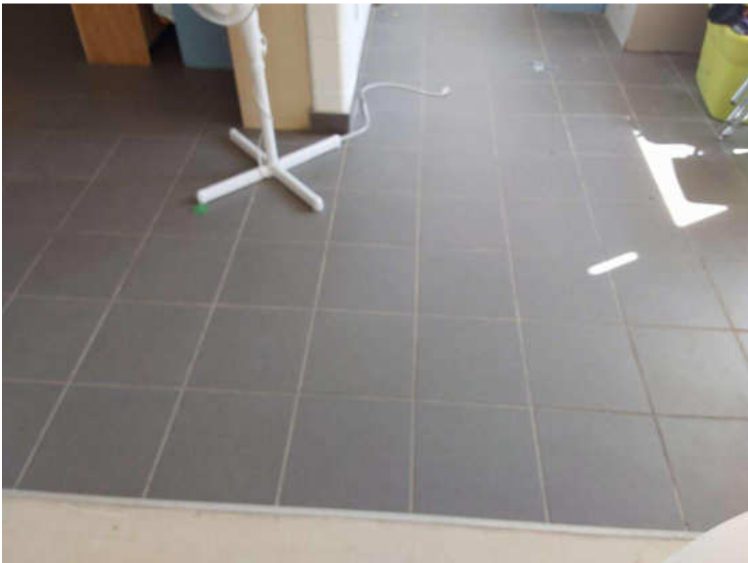
V9500 (Presumed Asbestos), Floor, Mortar, Room 2 (Location #: 8) Renovated space
