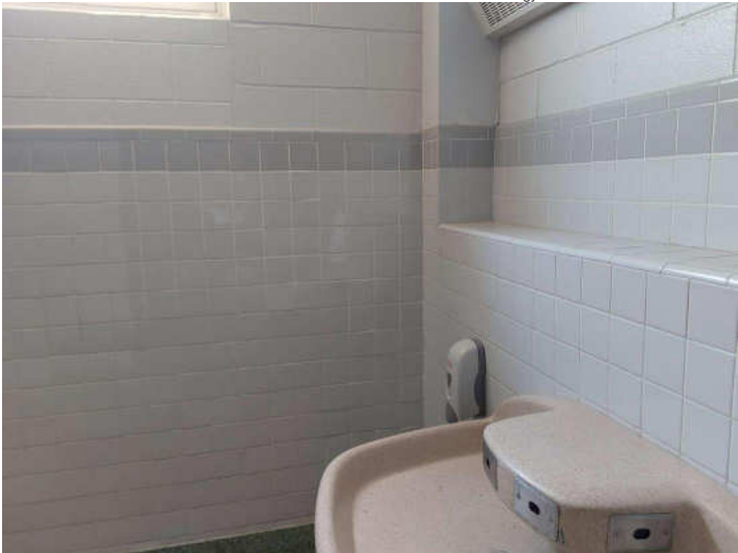
V9500 (Presumed Asbestos), Wall, Mortar, Men's Washroom (Boys) (Location #: 12)
