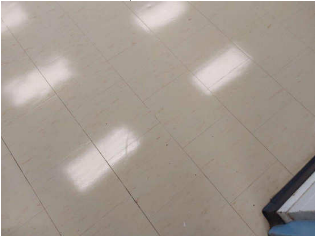
V0003 (Confirmed Asbestos), 12 x 12 tan with white and brown flecks, Floor, Vinyl Floor Tile and Mastic, Classroom 109 (Location #: 29) Mastic is presumed to contain asbestos
