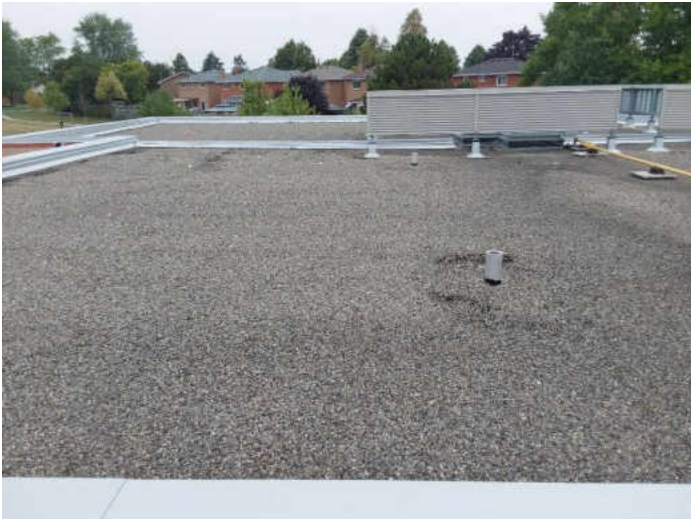
S0009A (Confirmed Asbestos), Other, Roofing material, Roof2 (Location #: 55)
