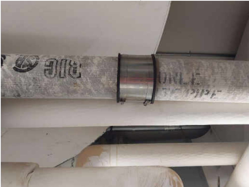
V9000 (Confirmed Asbestos), Piping, Rainwater Leader, Cement Product, Boiler Room (Location #: 44) Transite pipe
