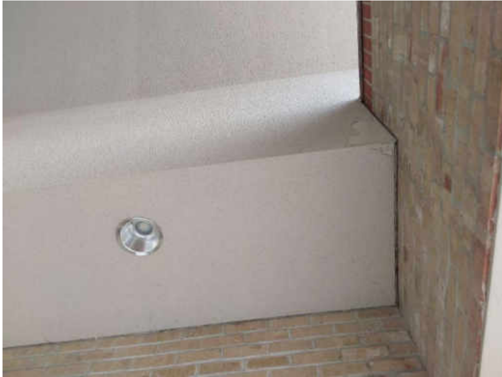
V9500 (Presumed Asbestos), Other, Cement Product, Exterior (Location #: 1) Transite panels above main entrance
