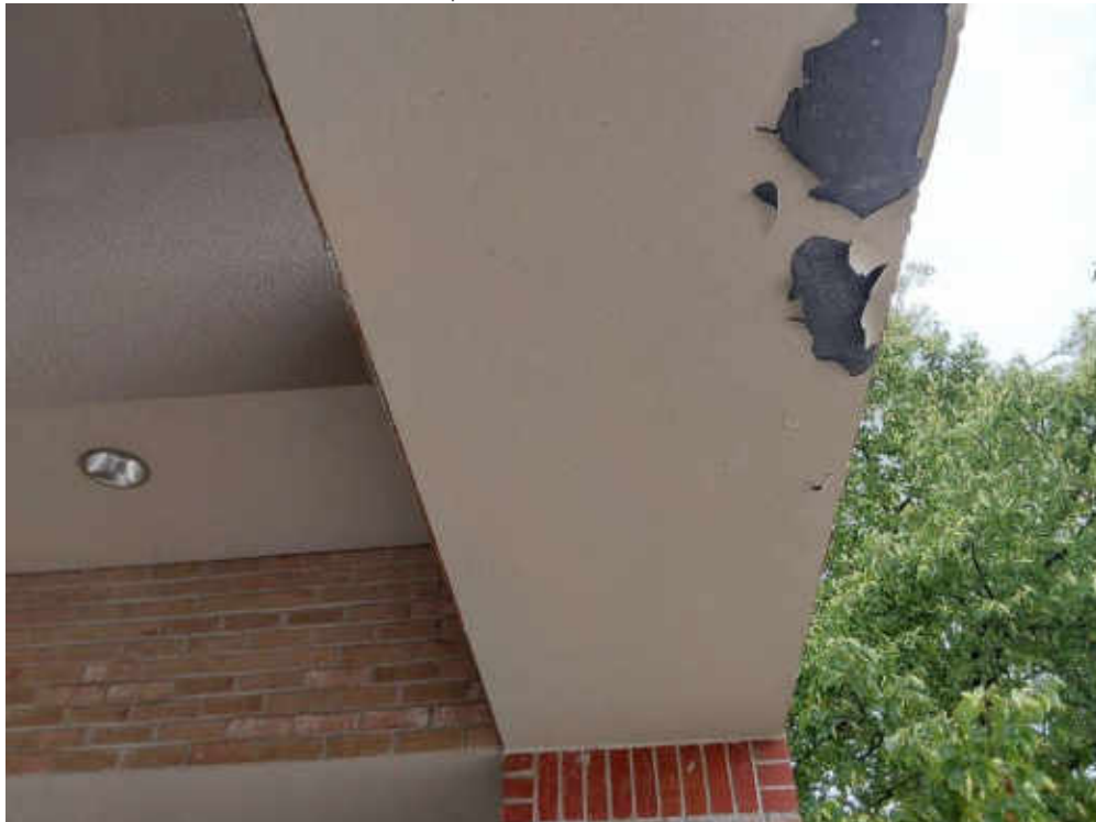
V9500 (Presumed Asbestos), Other, Cement Product, Exterior (Location #: 1) Transite panels above main entrance
