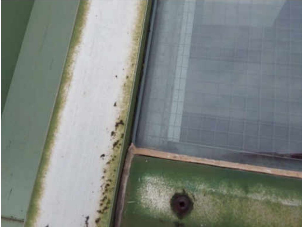
S0017A (Confirmed Asbestos), Butyl Sealant, Other, Window Liner, Caulking, Roof 1 (Location #: 54) On Atrium and Chapel window panes and frames.
