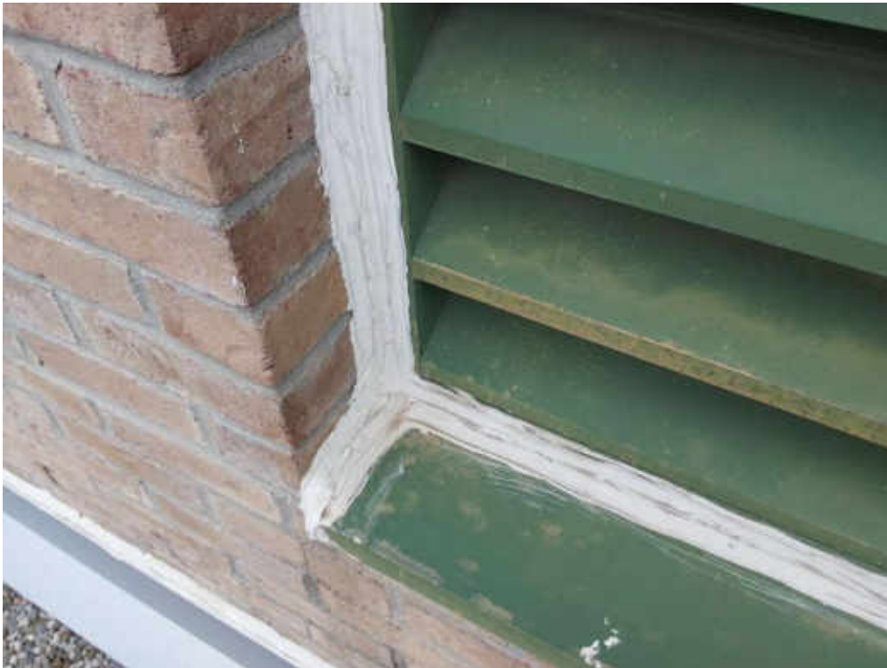
S0006A (Confirmed Asbestos), Black caulking on roof louvers, Other, Caulking, Roof 1 (Location #: 54) Beneath new white caulking on roof louvers, b126740 - 2016 - 0002
