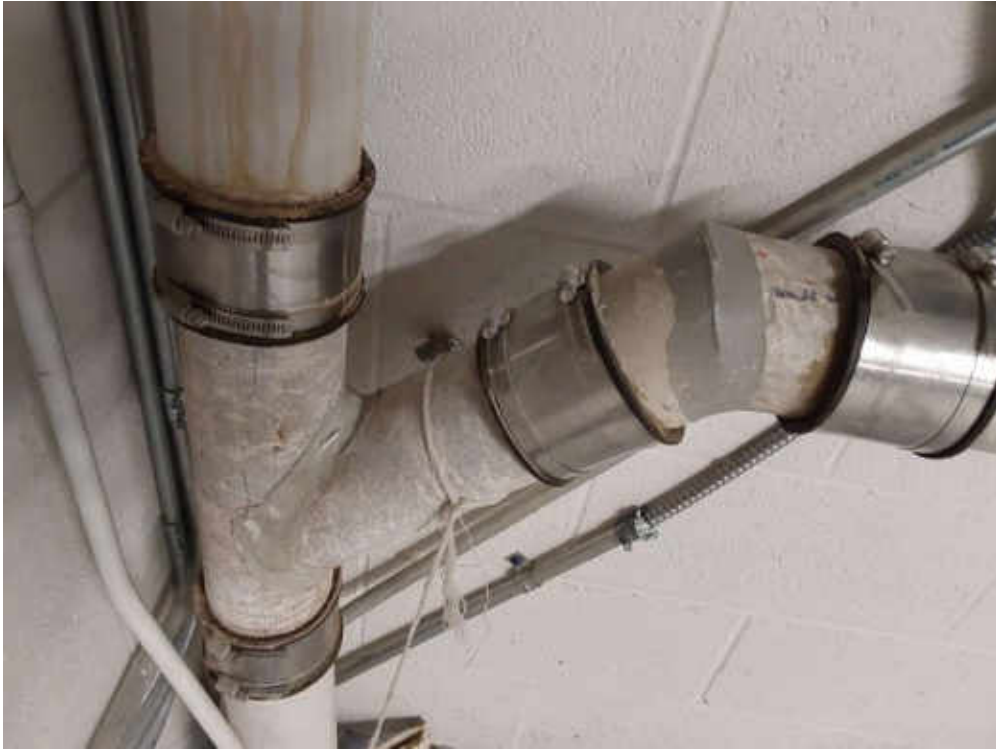
S0002A (Confirmed Asbestos), Cementitious adhesive, Other, Adhesive/mastic, Boiler Room (Location #: 44) On Transite rainwater leaders
