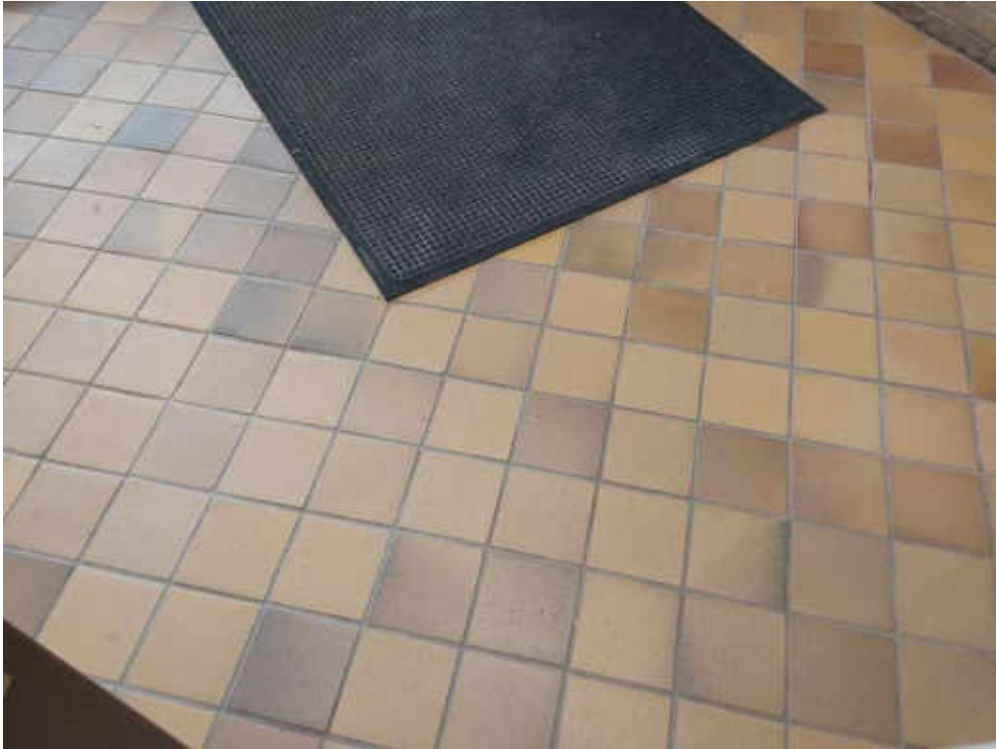
V9500 (Presumed Asbestos), Floor, All, Mortar, Vestibule (Location #: 2)
