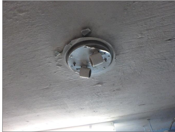
Asbestos-containing heat shield.
