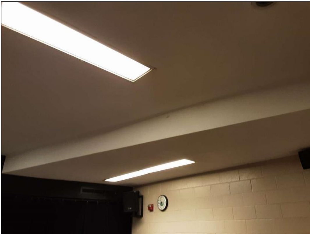
S0004A - (Confirmed Asbestos) Ceiling, Texture Coat, 102 (Location #: 1000)
