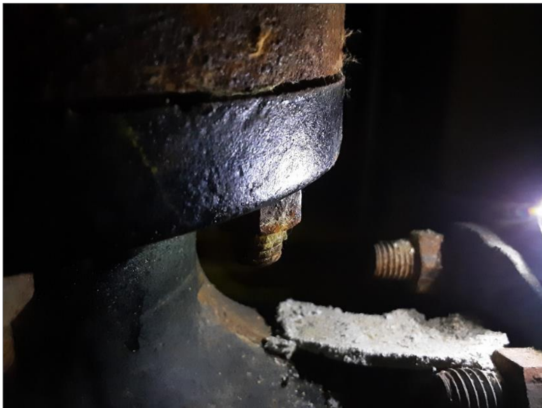
Damaged asbestos-containing piping cement insulation present on elbow and debris in Room 198 (Location #1960).
