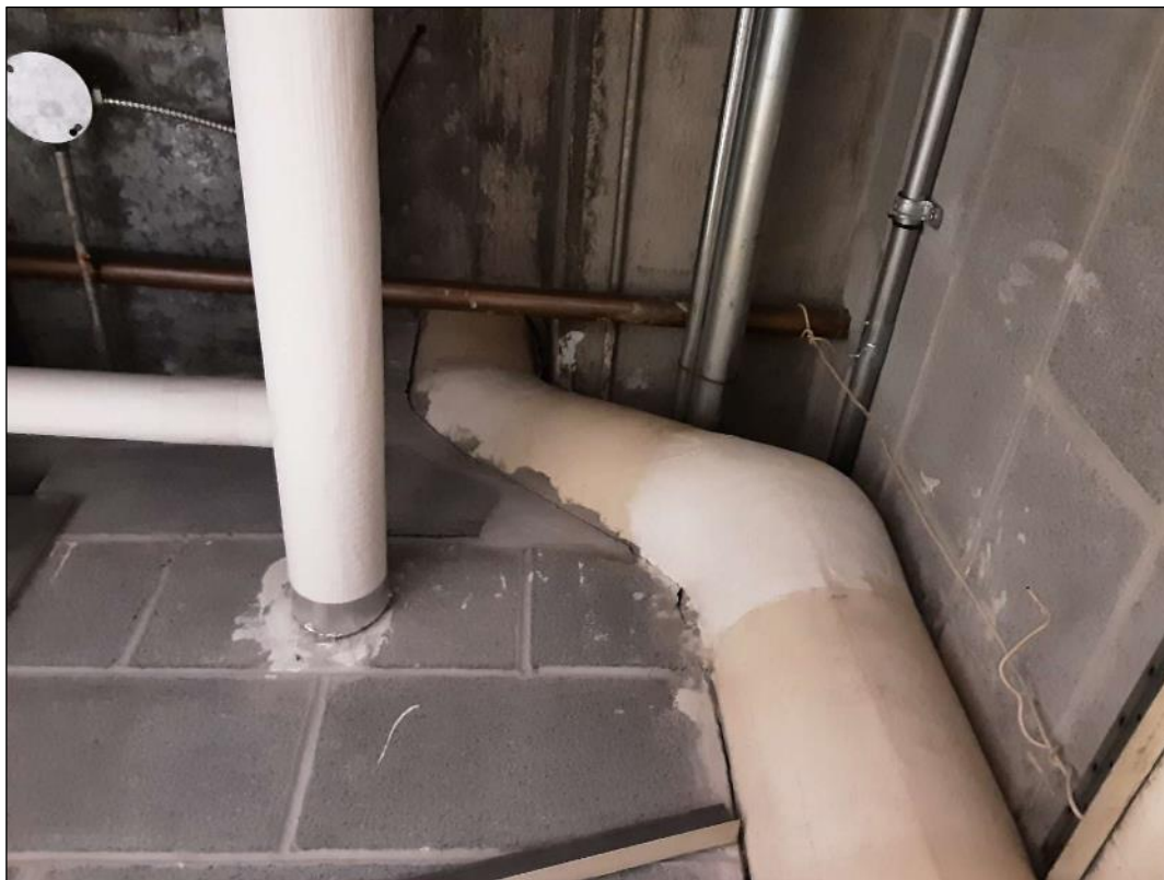
V0006 - (Confirmed Asbestos) Piping, Parging Cement, 120A (Location #: 1433)
