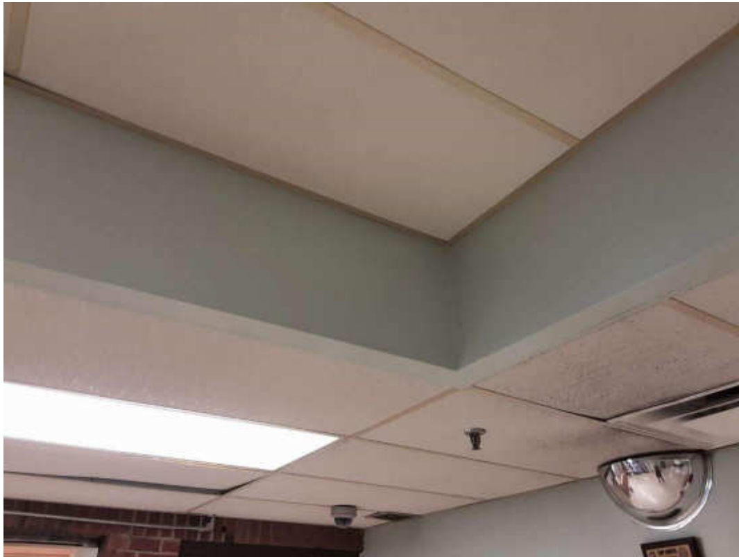
V0009 (confirmed Asbestos), Ceiling, Drywall on bulkhead, Lobby (Location #: 4)
