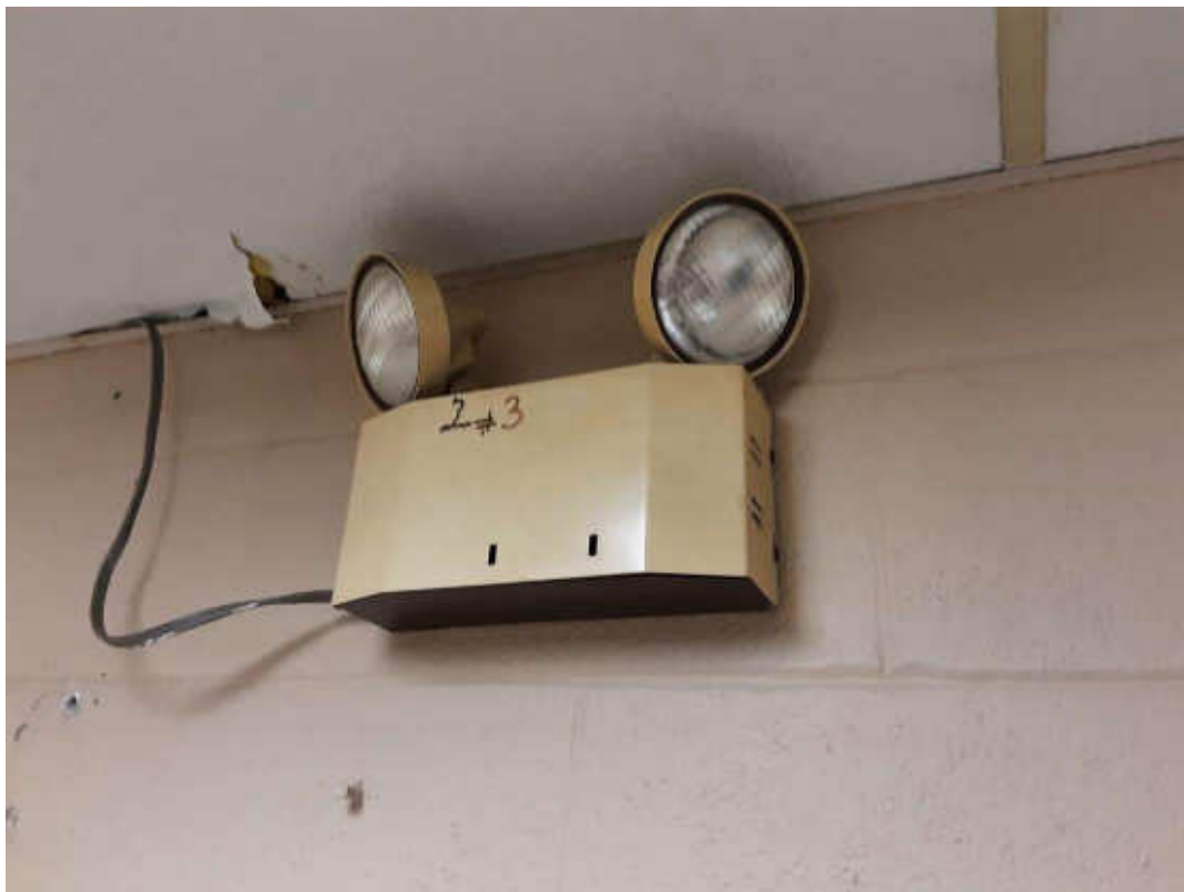
Pb Products, West Corridor (Location #: 56)
