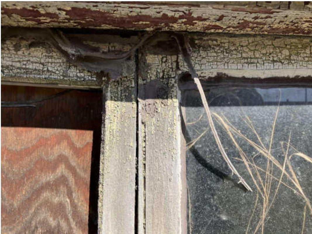
S0100C (None), Grey caulking on exterior windows, Exterior (Old House) (Location #: 180)
