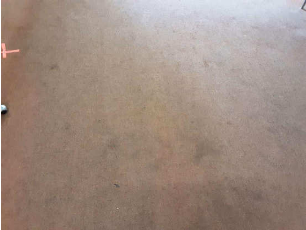
S0039A (None), Floor, Adhesive/mastic, Storage (Location #: 118)
