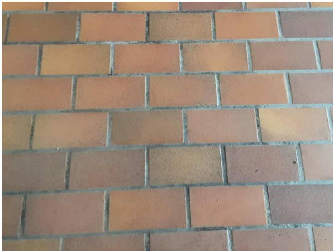
S0079A (Confirmed Asbestos), Floor, Thinset below 2" x 6" red faux brick ceramic tile, Vestibule (Location #: 116)
