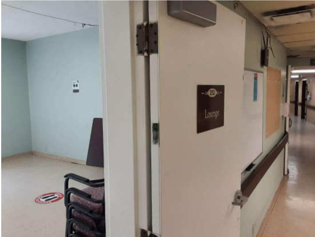
V0084 (None), Other, Fire Door, Corrugated Paper, Lounge (Location #: 11)
