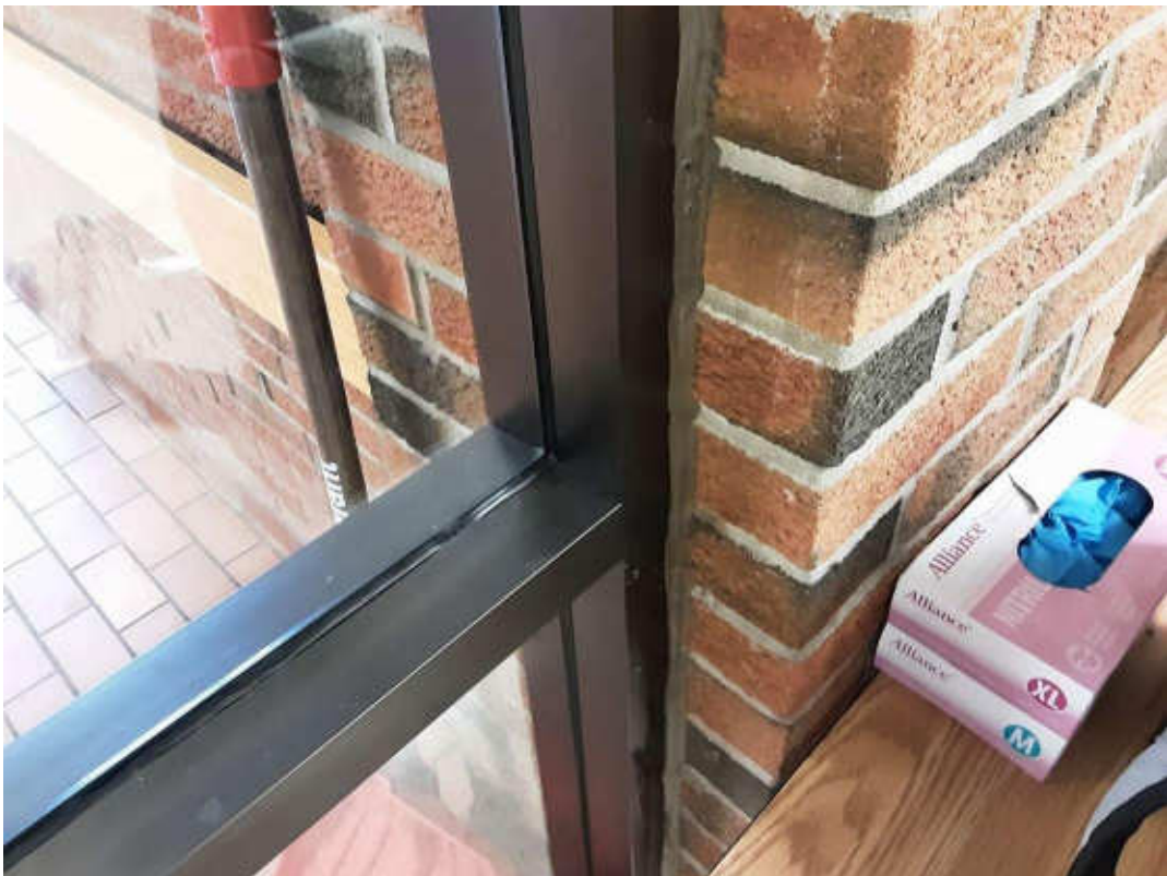
S0005A (None), Other, Door, Caulking, Lobby (Location #: 4)
