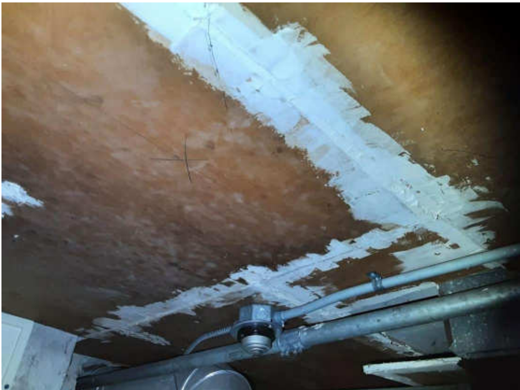
S0040A (Confirmed Asbestos), Ceiling, Drywall and joint compound, Old House - Basement (Location #: 135)
