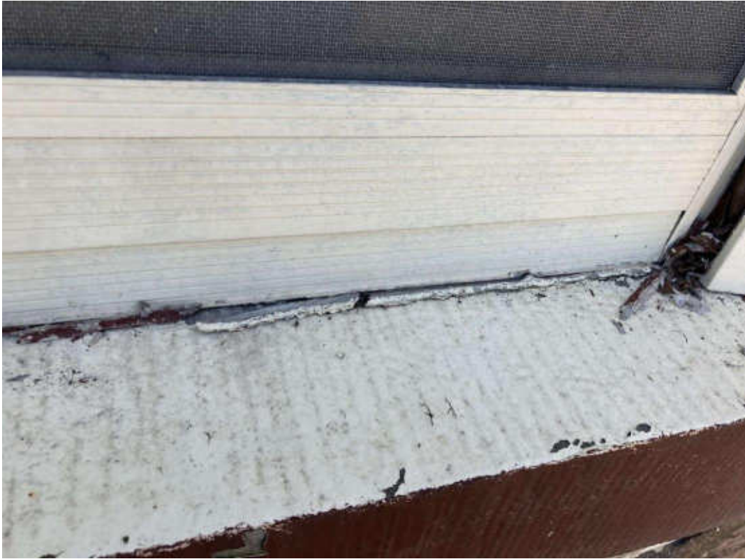
S0099C (Confirmed Asbestos), Light grey window caulking, Other, Caulking, Exterior (Old House) (Location #: 180)
