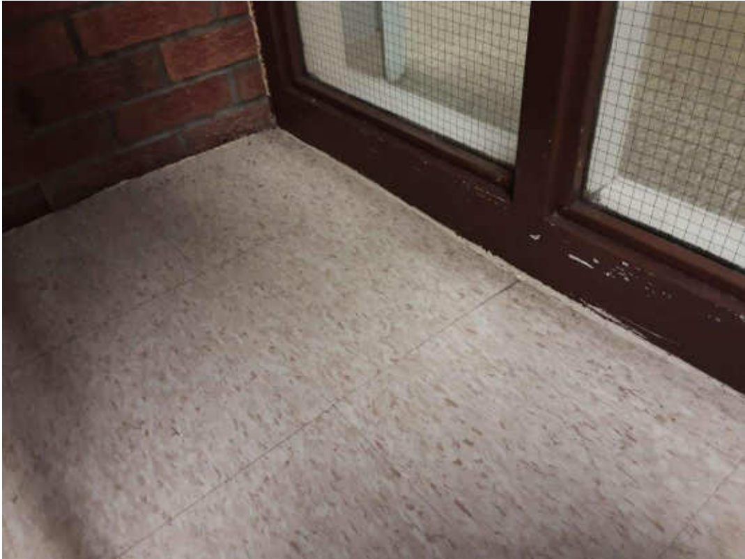
S0006A (None), Wall, Base, Caulking, Lobby (Location #: 4)
