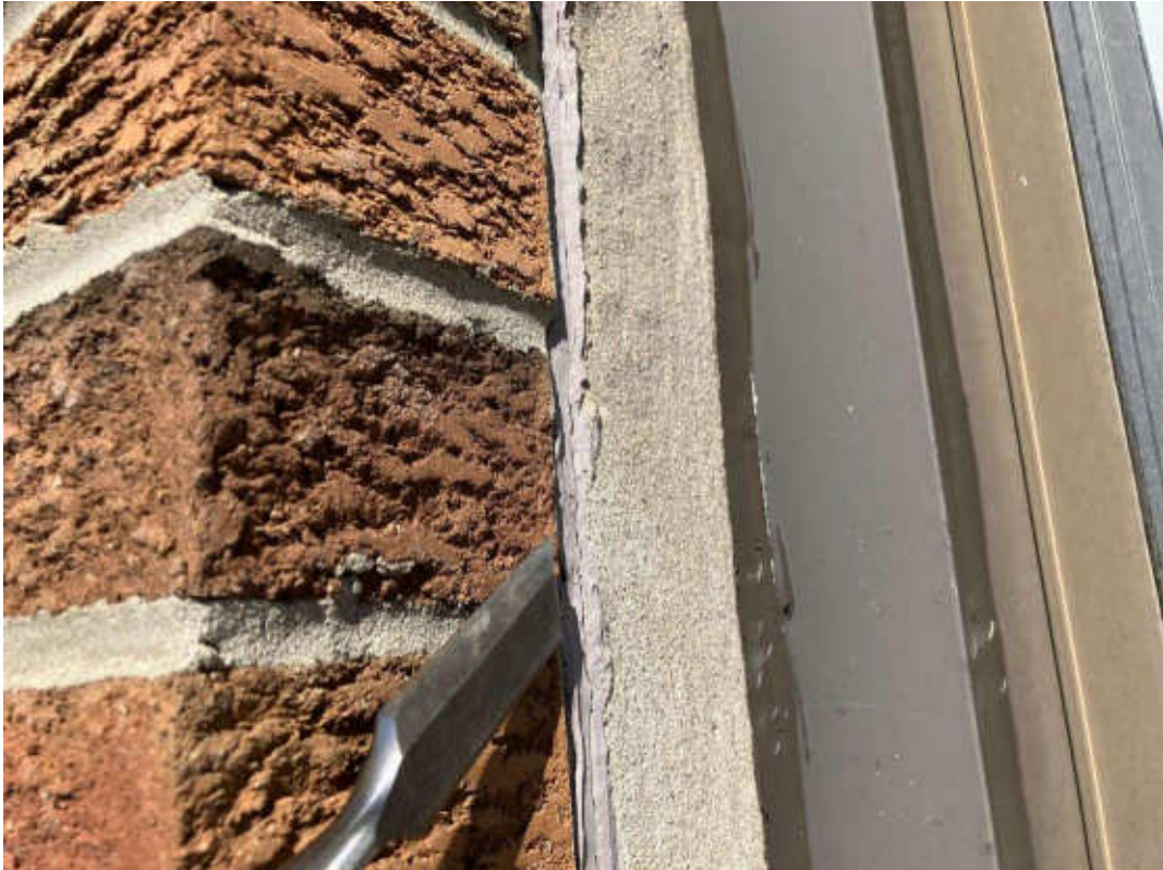
S0101C (None), Light grey caulking on exterior windows, Exterior (West Wing) (Location #: 181)
