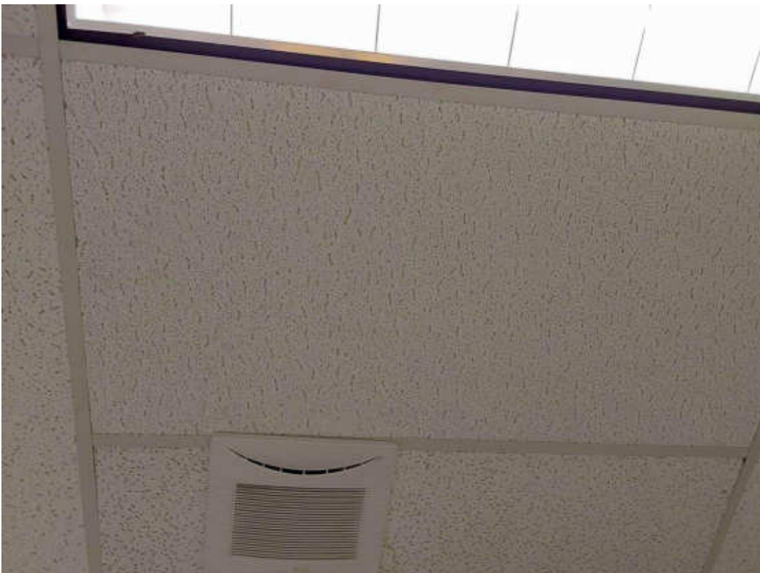
V0000 (None), 24" x 48" pinhole and large fleck, Ceiling, Ceiling Tiles (lay-in), Men's Washroom (Location #: 1) Date stamp 10/08/01
