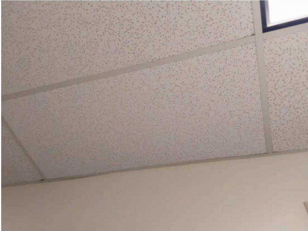
V0000 (None), 24" x 48" pinhole and small sparse fleck, Ceiling, Ceiling Tiles (lay-in), Office Area And Corridors (Location #: 3) Date stamp 10/02/10
