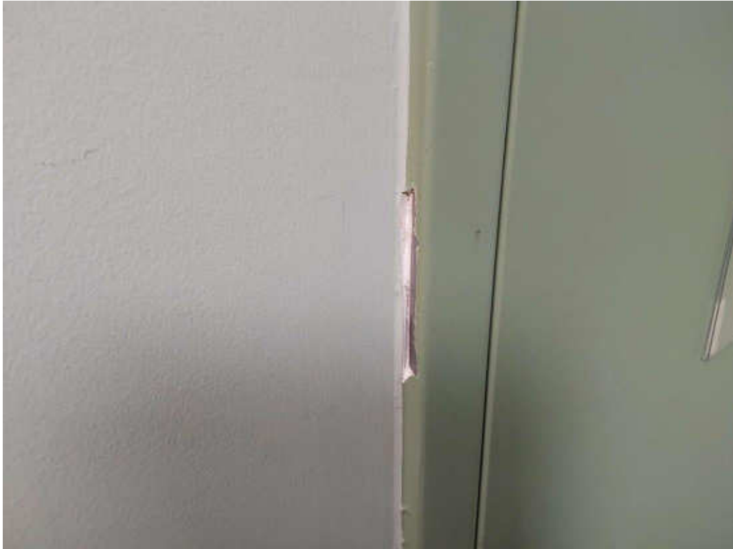
S0007A (None), White caulking on door frame, Other, Caulking, Women's Washroom (Location #: 2)
