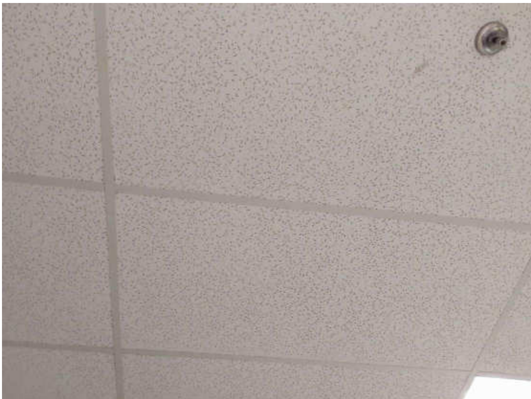
S0004B (None), 24" x 48" pinhole and small fleck, Ceiling, Ceiling Tiles (lay-in), Men's Washroom (Location #: 1)
