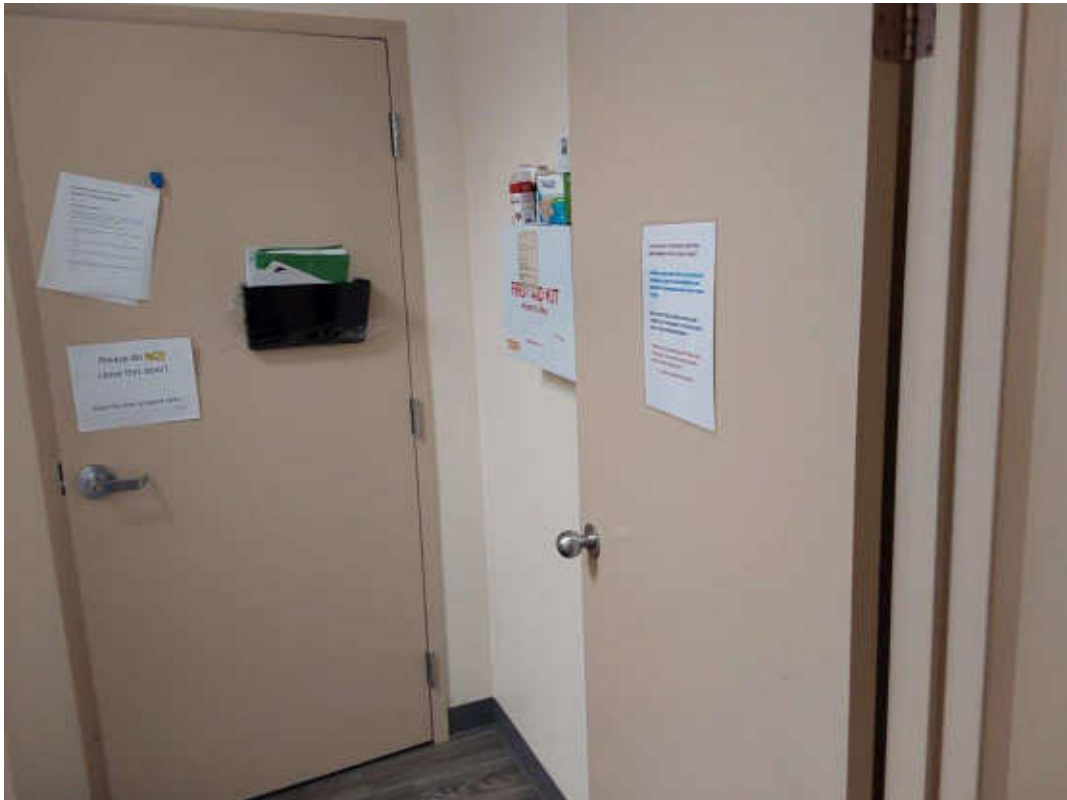
L0004(Lead, None), Tan paint on doors, Wall, Office Area and Corridors (Location #: 3)
