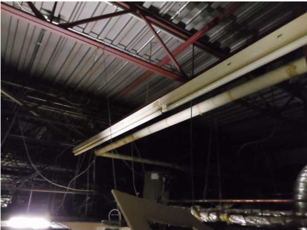
PCB, V9500(Presumed), LIGHT BALLASTS, T12 fixtures above ceiling, Men's Washroom (Location #: 1)
