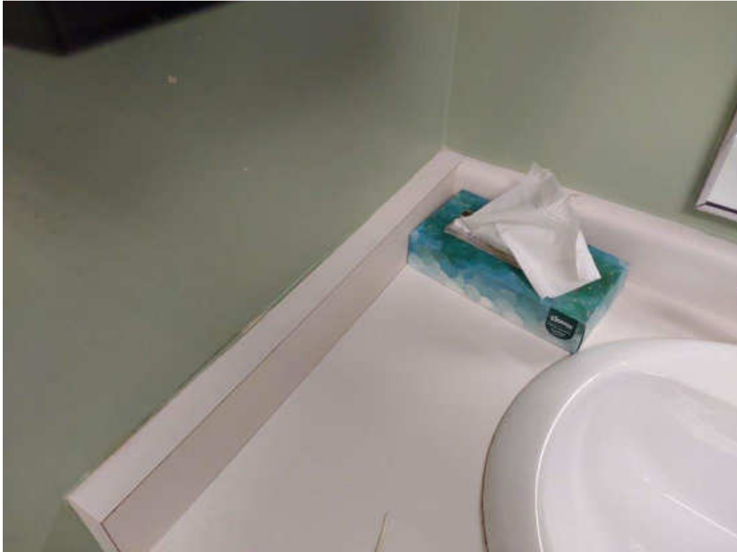
S0005B (None), White caulking on sink shelf, Other, Caulking, Men's Washroom (Location #: 1)
