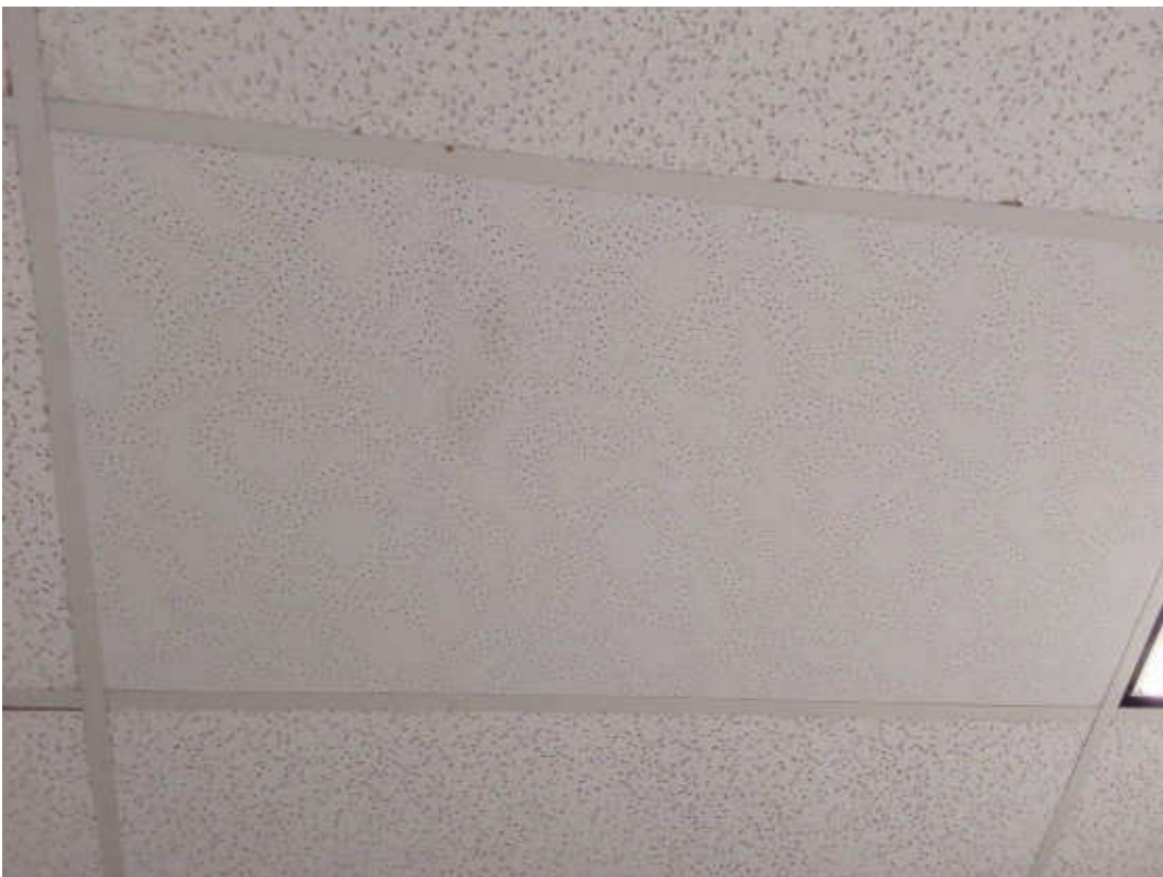
V0000 (None), 24" x 48" small and large pinhole, Ceiling, Ceiling Tiles (lay-in), Women's Washroom (Location #: 2) Date stamp 08/11/98
