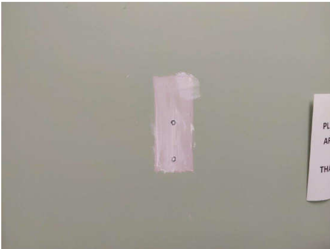
L0003(Lead, None), Lavender paint on drywall beneath green paint, Wall, Women's Washroom (Location #: 2)
