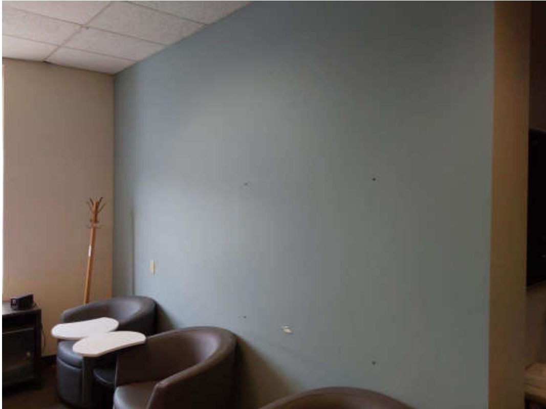
L0006(Lead, None), Blue paint on drywall, Wall, Office Area and Corridors (Location #: 3)
