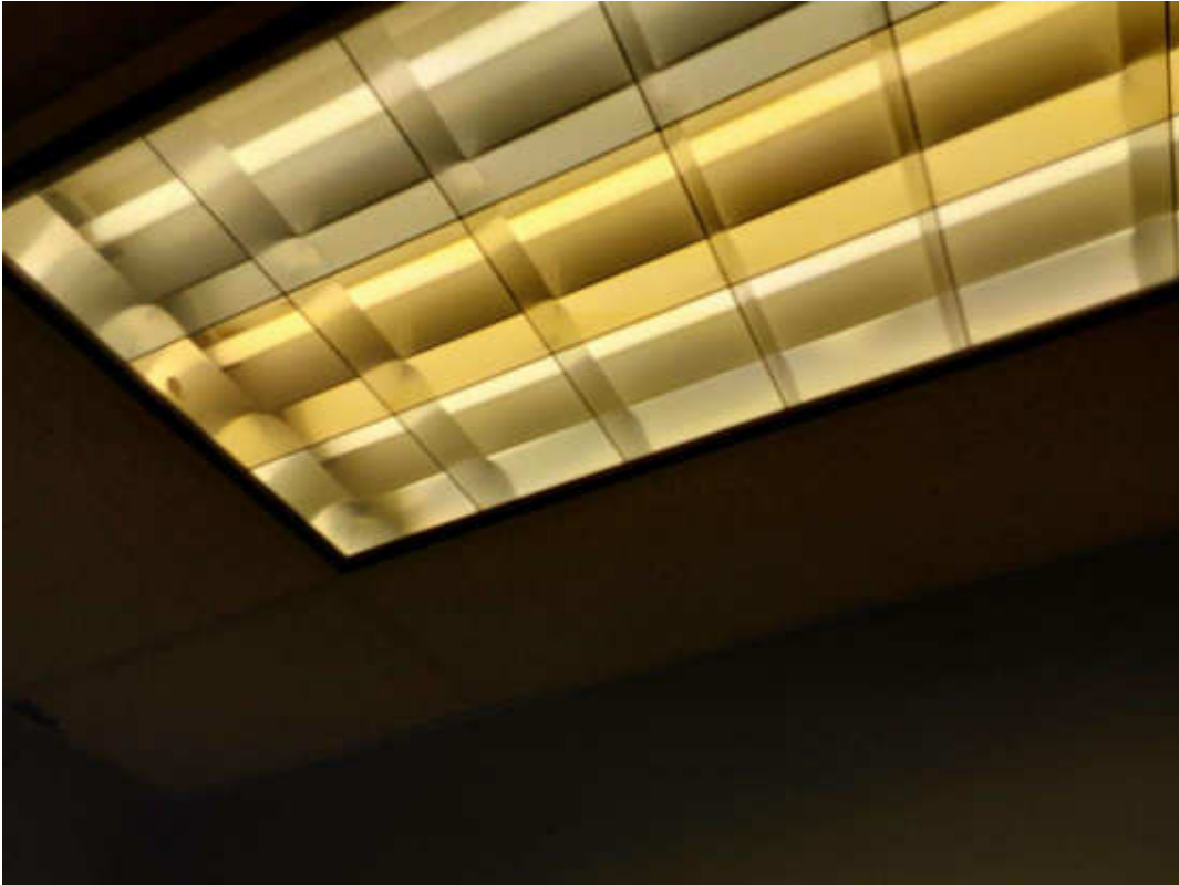
Mercury, V9000(Yes), LIGHT FIXTURE, T8 fixtures, Men's Washroom (Location #: 1)
