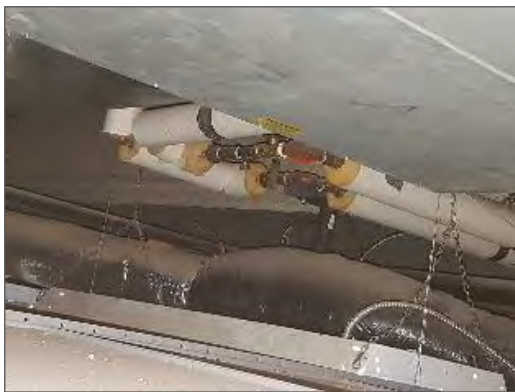
Photo 1 – Non-asbestos fibreglass pipe insulation on heating system pipes above lay-in ceiling tiles in room 104.
