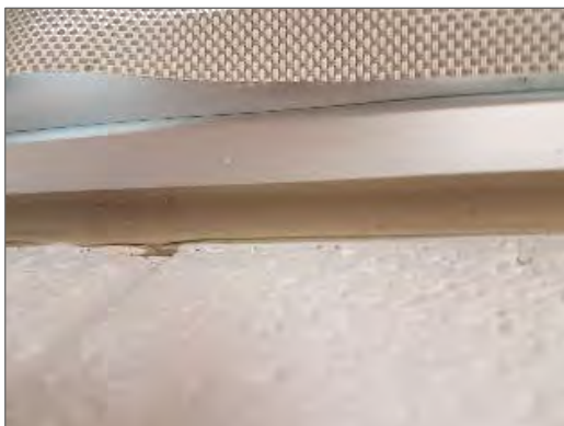
Photo 7 – Tan coloured caulking in Room 104 on window frame. Does not contain asbestos.
