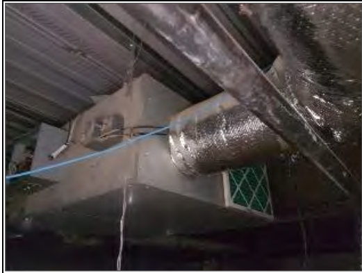
Photo 4 – Uninsulated heating equipment above lay-in ceiling tiles in room 104.
