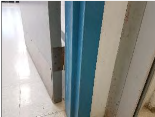
Photo 10 – Blue on metal door frame.
