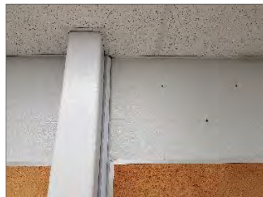
Photo 9 – Pale blue paint on metal beam.
