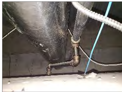
Photo 2 – Uninsulated pipe above lay-in ceiling tiles in room 104.
