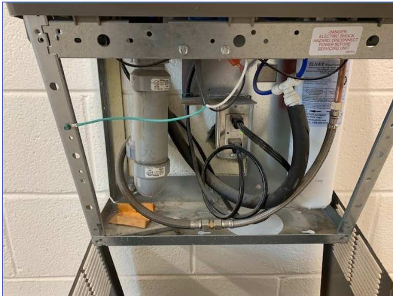
Figure 2 Sample power installation of GFI outlet
