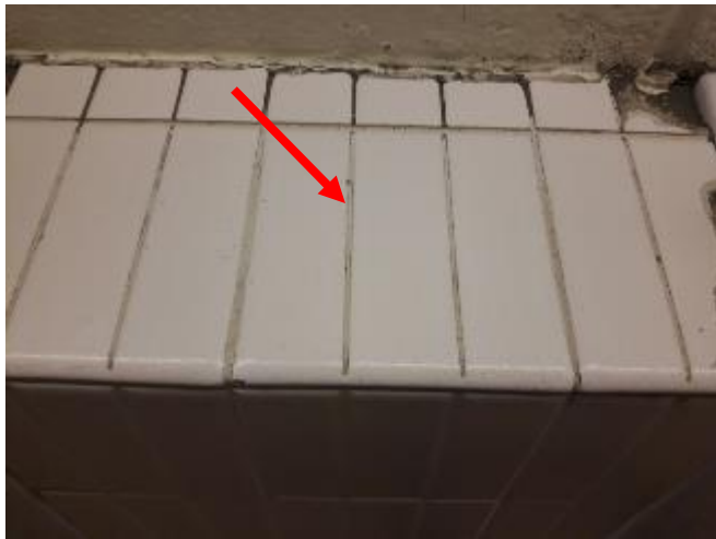
Photo 3: View of the non-asbestos containing mortar (see arrow) observed on beige tiles within Room 122.
