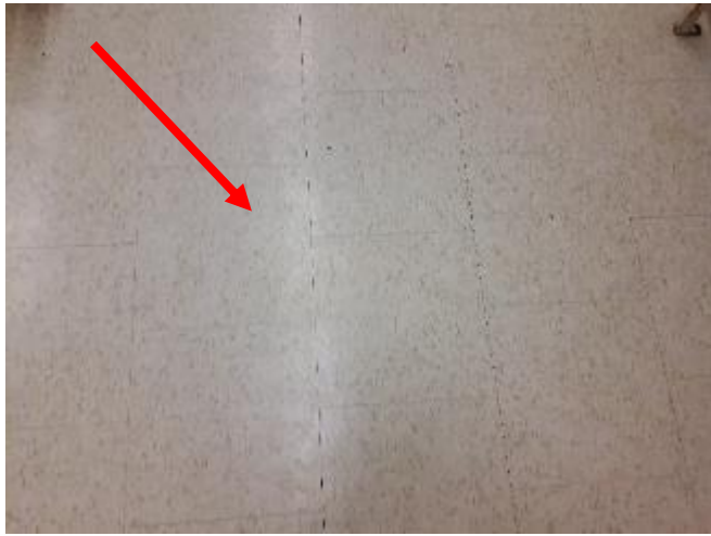
Photo 1: View of the asbestos containing 12"x12" light brown vinyl floor tiles (see arrow) observed in Room 138.
