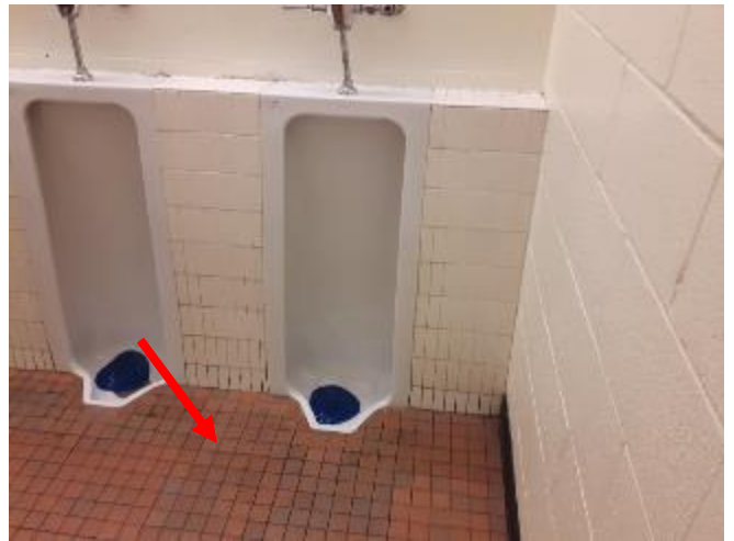
Photo 4: View of the non-asbestos containing mortar (see arrow) observed on terracotta tiles within Room 122.
