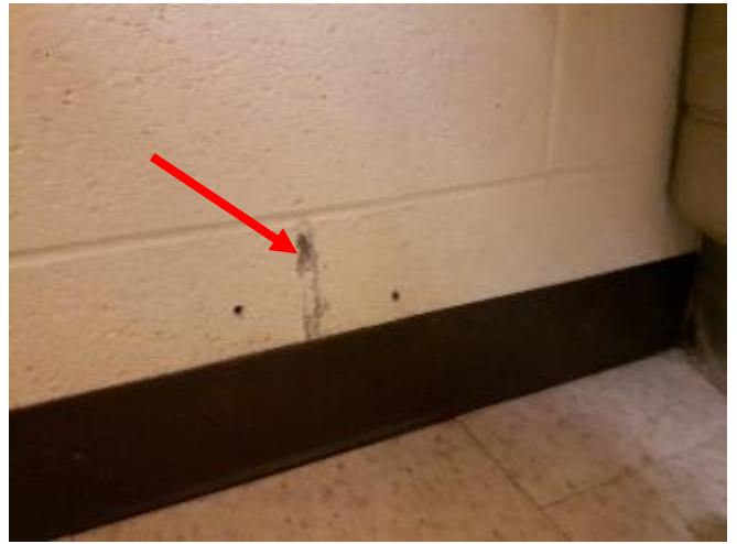
Photo 2: View of the non-asbestos containing concrete block mortar (see arrow) observed in Room 138.
